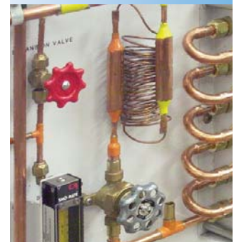
A/C, Refrigeration & Boilers
