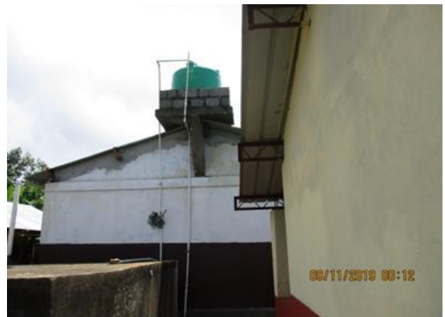
Cistern (water tower) to supply water to restrooms
