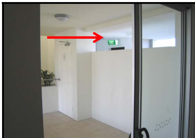
Figure 4 – View from inside the unit showing entry door and opening to the “courtyard”.
