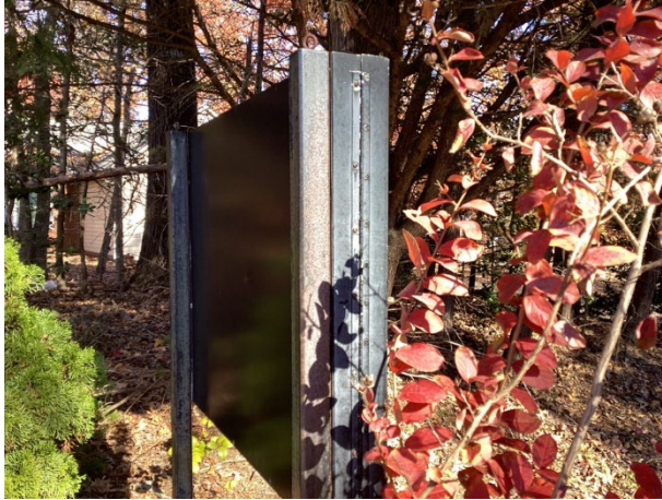
Frame finish deterioration and rust
