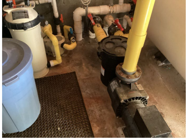
Pool mechanical equipment
