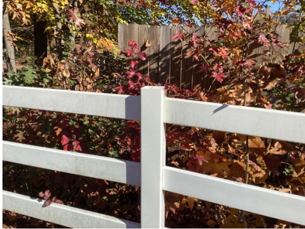
Missing post cap
