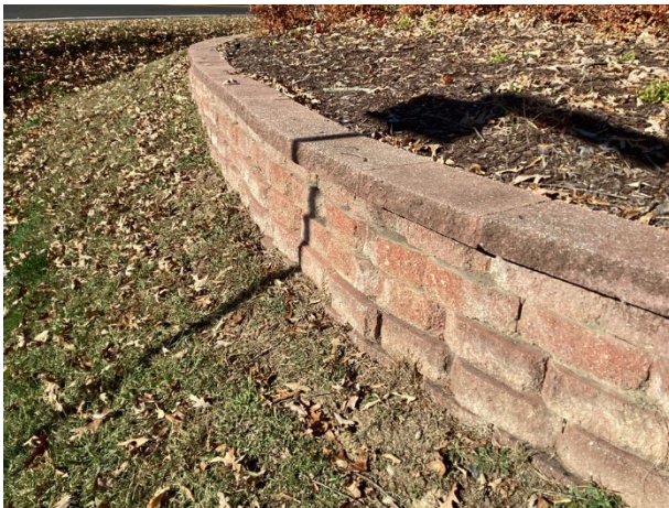
Minor retaining wall movement
