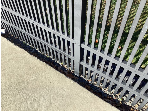
Fence finish deterioration
