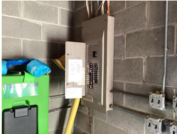
Electrical system main panel at pool house
