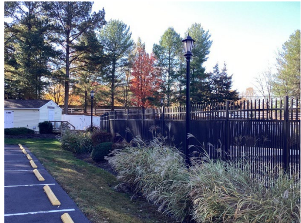
Light poles and fixtures
