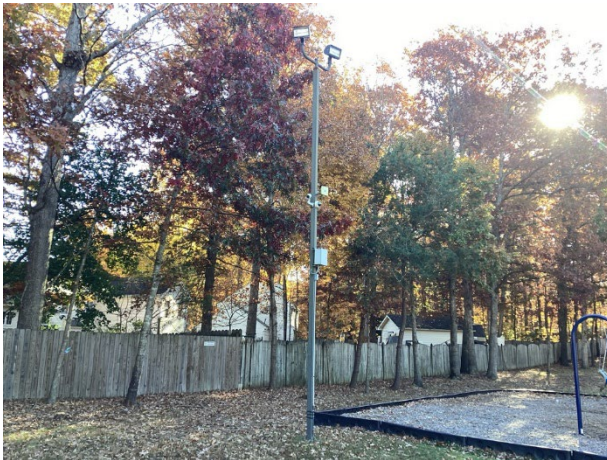
Light pole and fixtures
