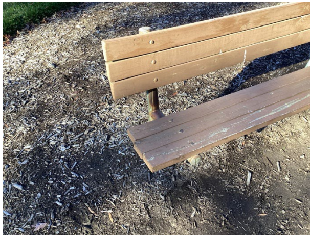
Finish deterioration and rust
