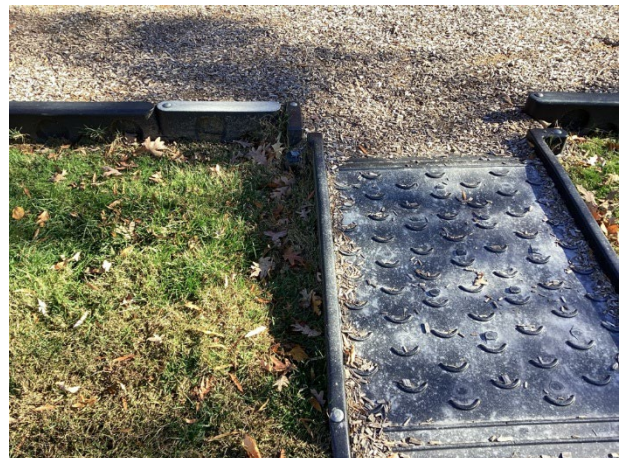
Border finish deterioration
