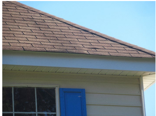
Shingle lift and wear
