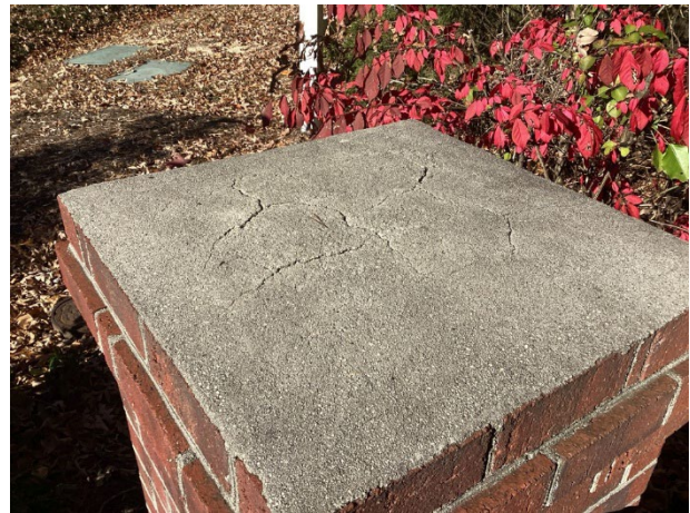
Cracks at concrete coping
