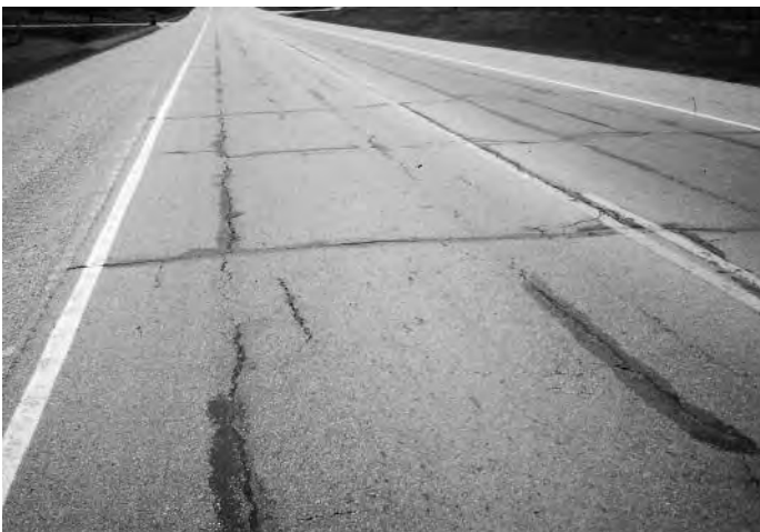
▼ Load-related cracks in wheel path.
