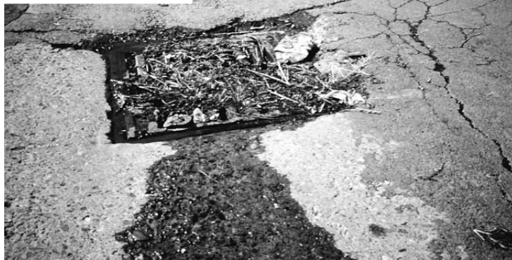
Pavement settlement causes ponding in this poor parking lot inlet.
