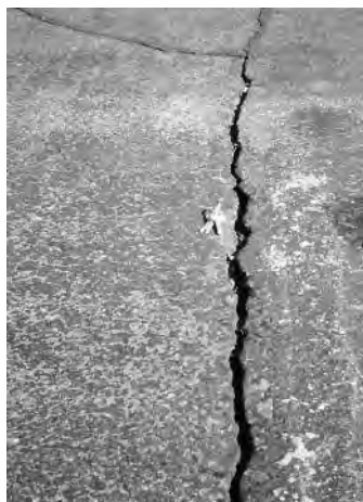
▲ Open crack – 1/2" or more in width.
