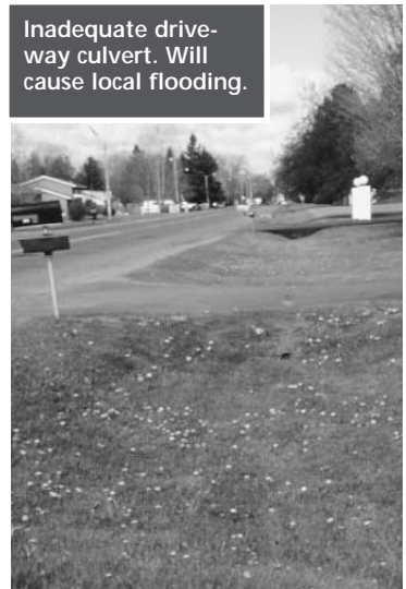
No ditch for extensive portion of roadway.
