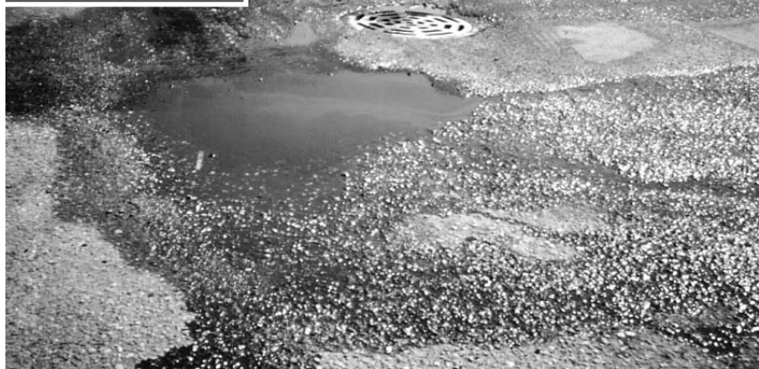
Clogged inlet causes flooding.
