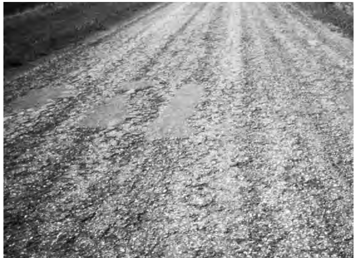
◀ Severe raveling and loss of surface material.
