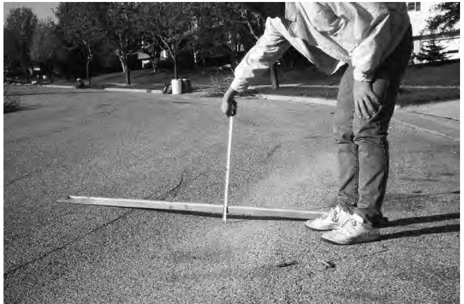
► Severe settling from utility trench.
