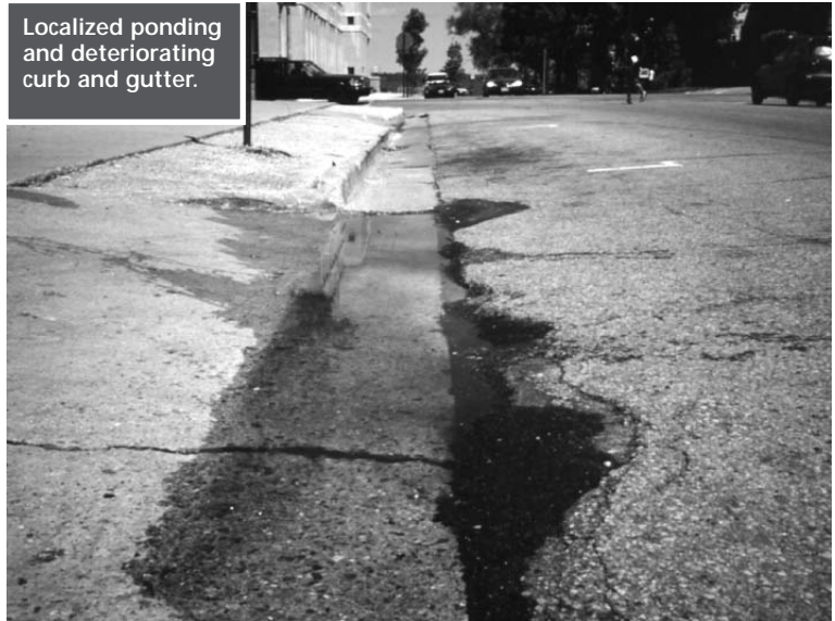
Clean drain and sewer to prevent localized flooding.
