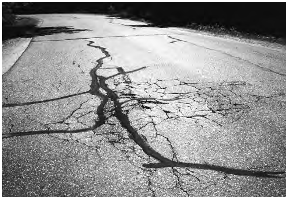
► Frost heave damage from spring break-up.
