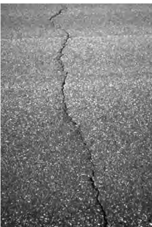
▲ Tight cracks less than 1/4" in width.
