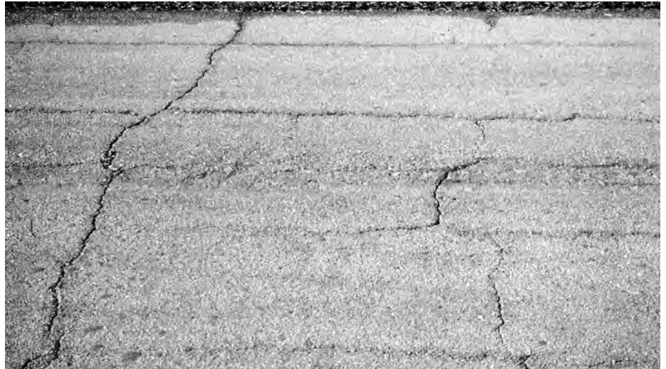
▼ Block cracking with open cracks.
