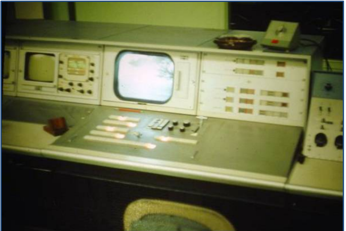
Another view of the video switcher.
