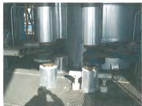
Above Valves in Silicon Plant in China
