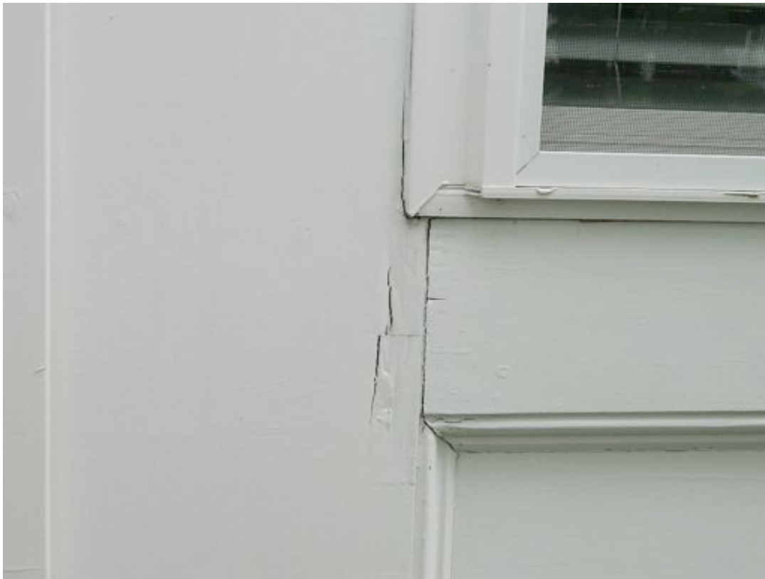
THE PANELS AROUND SOME WINDOWS ARE BEGINNING TO FAIL
