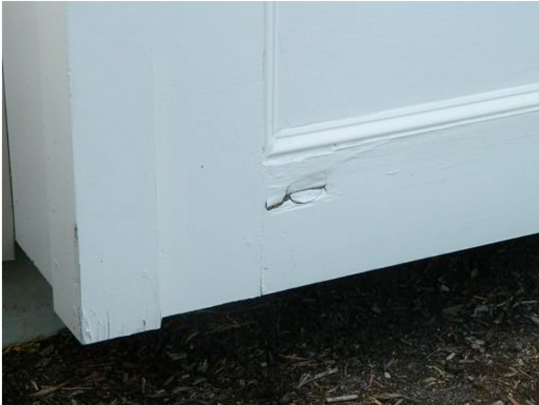
THE WINDOW "BUMP OUT" TRIM ROT IS LIKELY DUE TO INCOMPLETE INITIAL COATING
