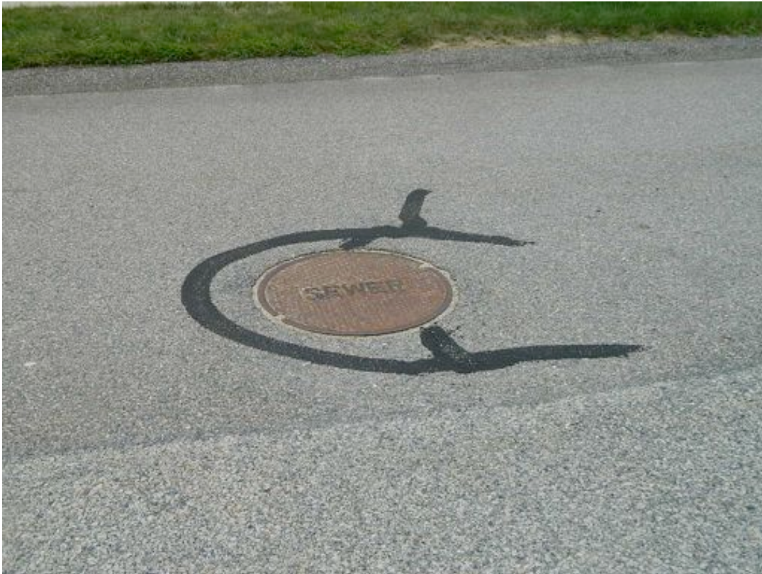
SOME SEALED CRACKING WAS NOTED AROUND ROADWAYS STRUCTURES
