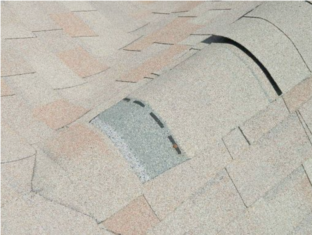
A FEW MISSING RIDGE CAP SHINGLES WERE NOTED (NOT WIDESPREAD)
