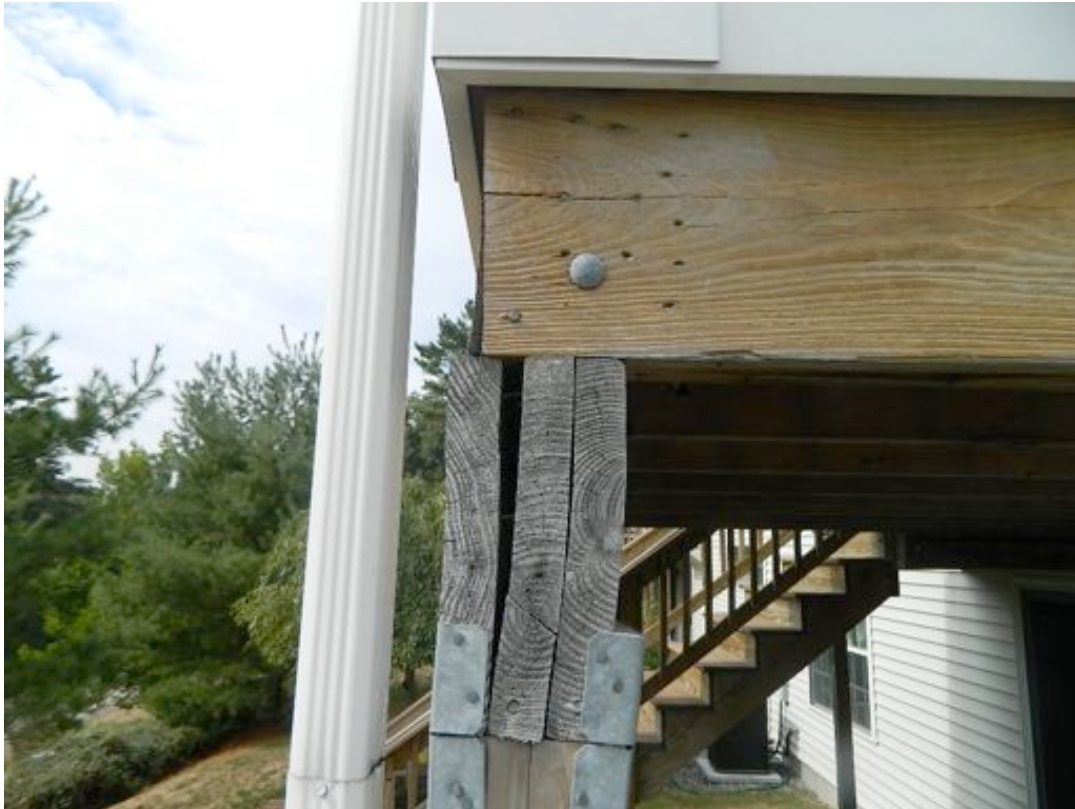
POOR ATTACHMENT AND FASTENER CHOICES HAS COMPROMISED SOME DECK FRAMING
