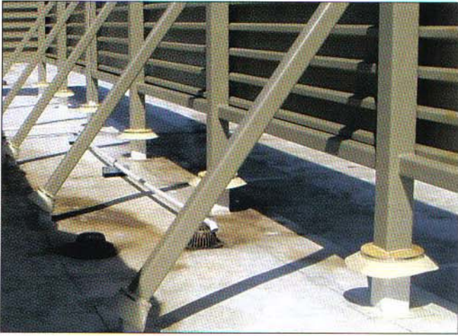
For equipment screens on the St. Luke's Outpatient Center rooftop (St. Louis, Missouri), the use of rubber retrofit storm collars rectified earlier problems with square tube steel columns.
