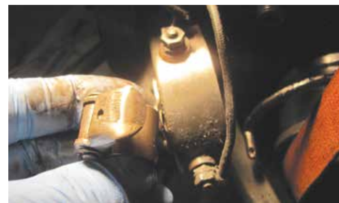
Anderson timer flapper showed considerable wear
