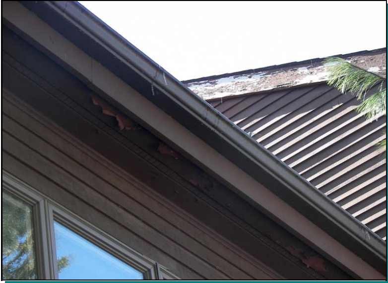
Chipped and blistered paint finish at wood soffit and fascia
