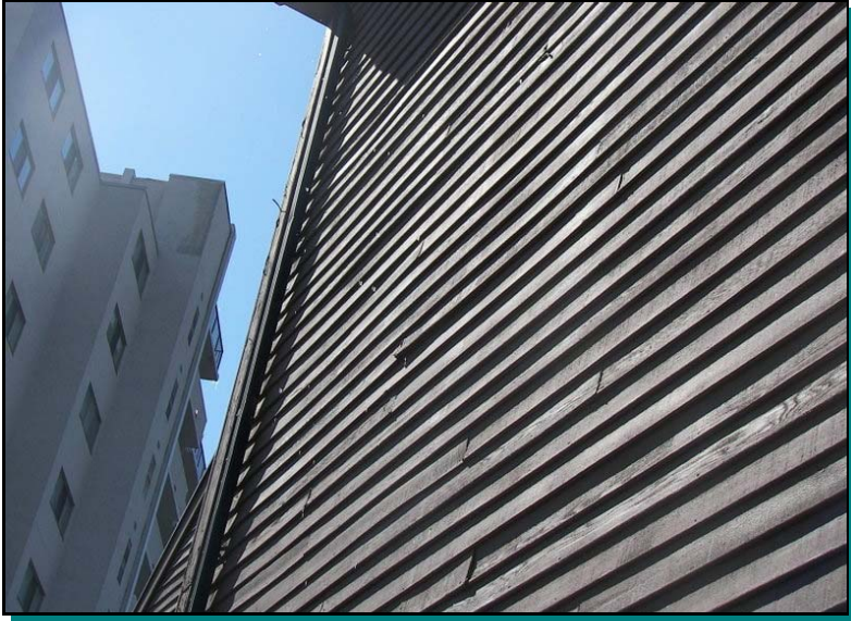
Loose and warped wood siding
