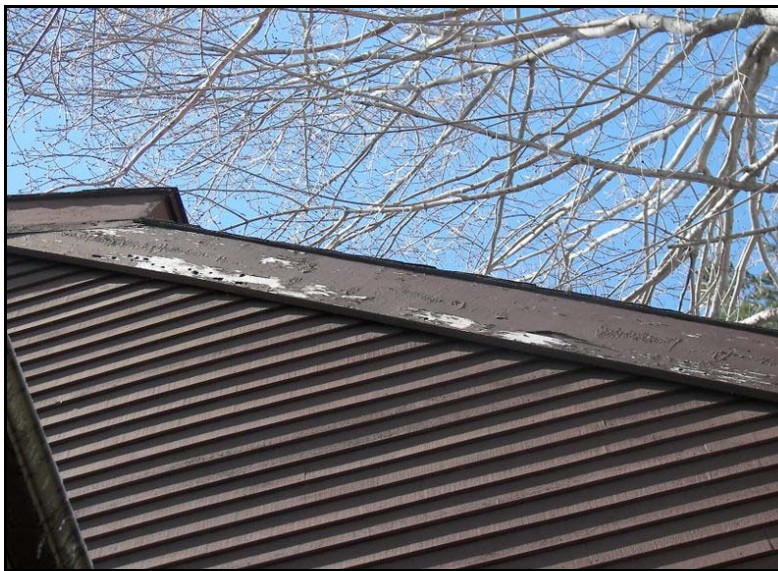
Chipped and blistered paint finish at wood fascia board
