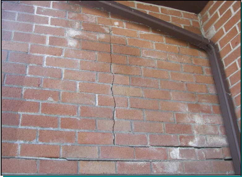
Severe cracks at brick masonry
