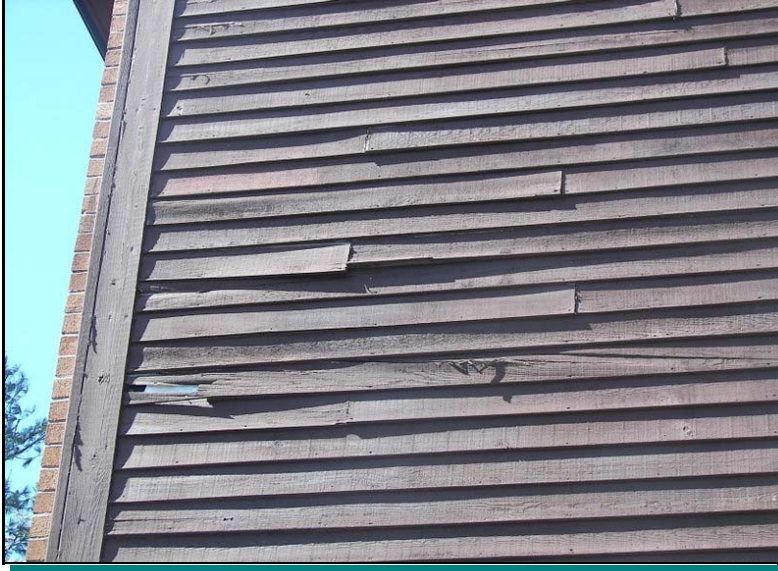
Cracked, rotted and bowed wood siding
