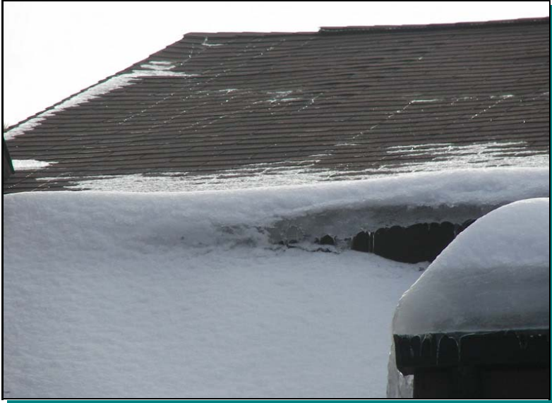
Roof exhibits shingle lift and sheathing deflection
