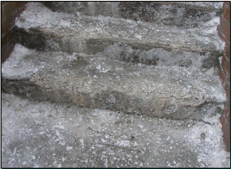
Spalls and deterioration at concrete steps
