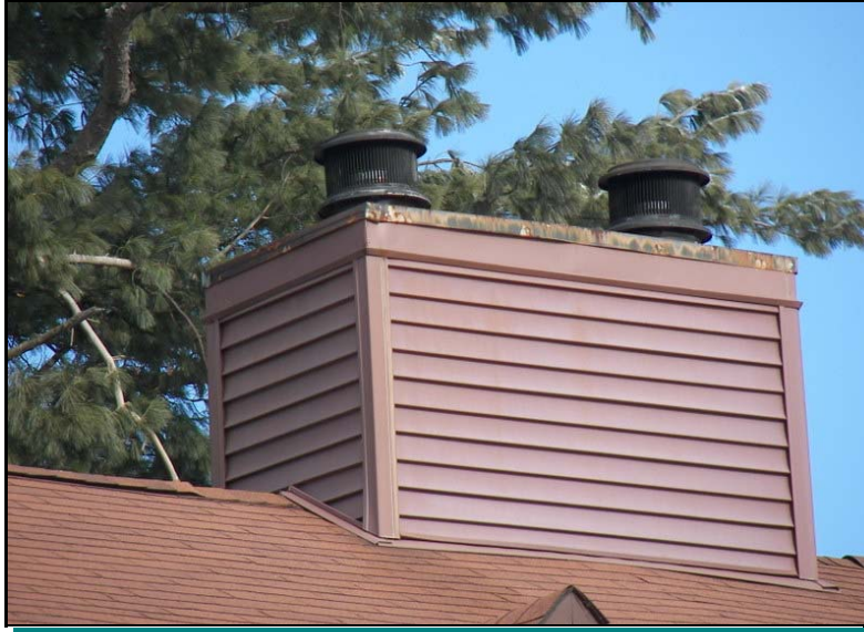
Rust and deterioration visible at metal chimney cap
