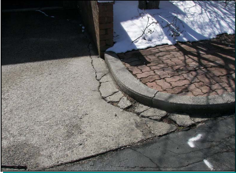
Cracks at concrete driveway
