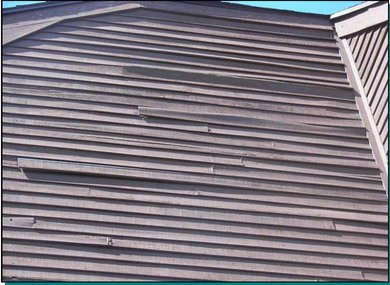
Loose, warped and bowed wood siding
