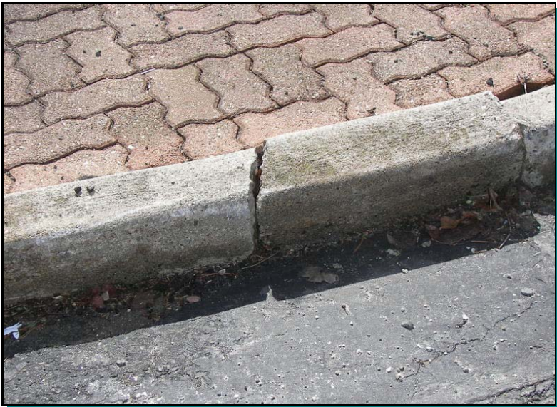
Cracked concrete curb
