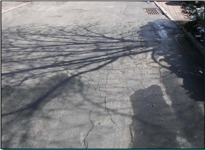
Alligator and surface cracks at asphalt pavement
