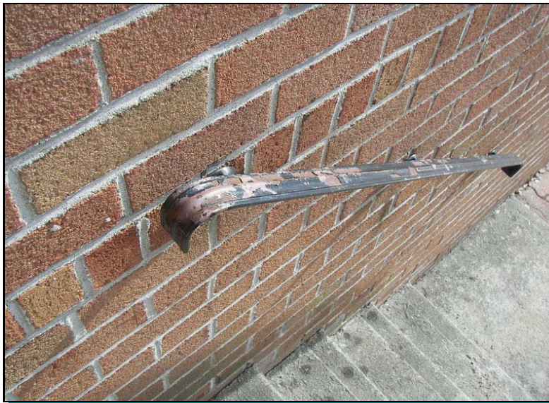
Paint deterioration at metal handrail
