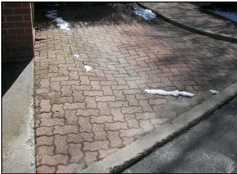
Rutting evident at brick paver parking area
