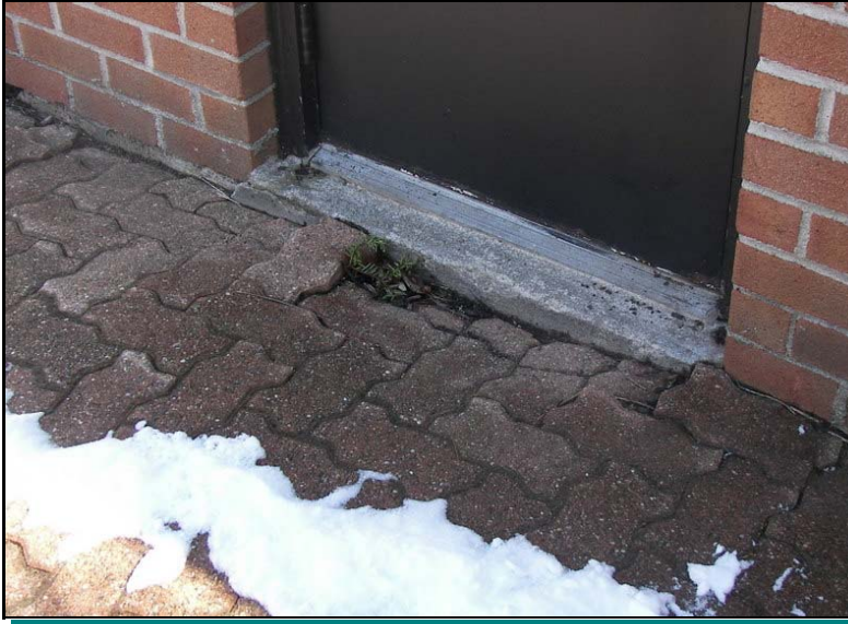
Example of settled and heaved brick pavers
