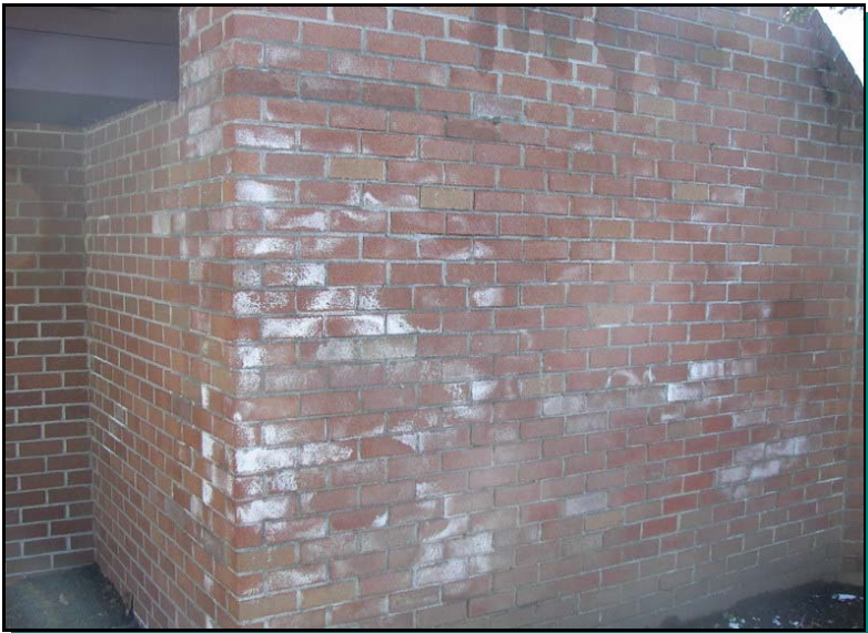
Efflorescence at brick masonry
