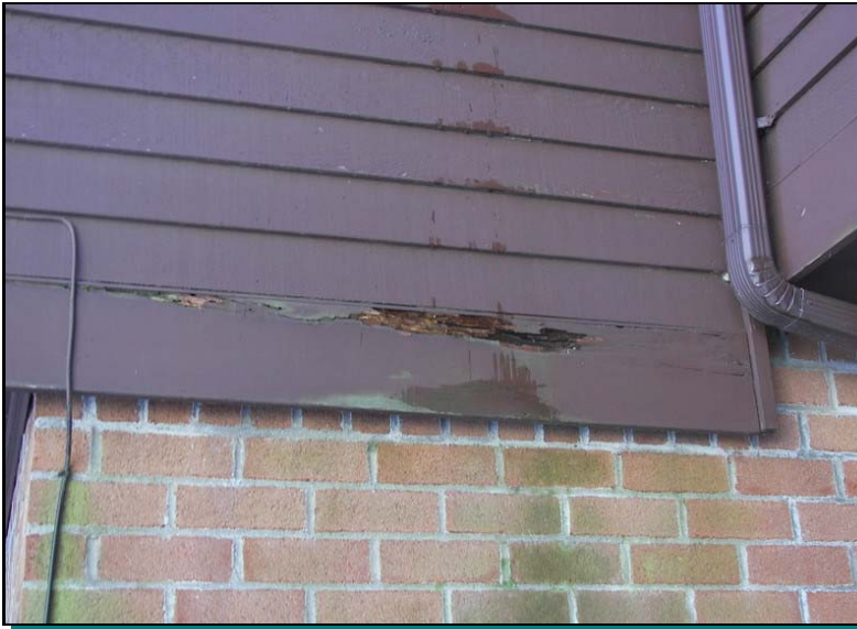
Wood rot evident at wood siding
