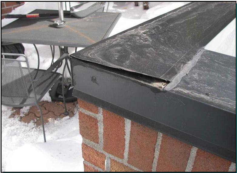
EDPM roof deterioration
