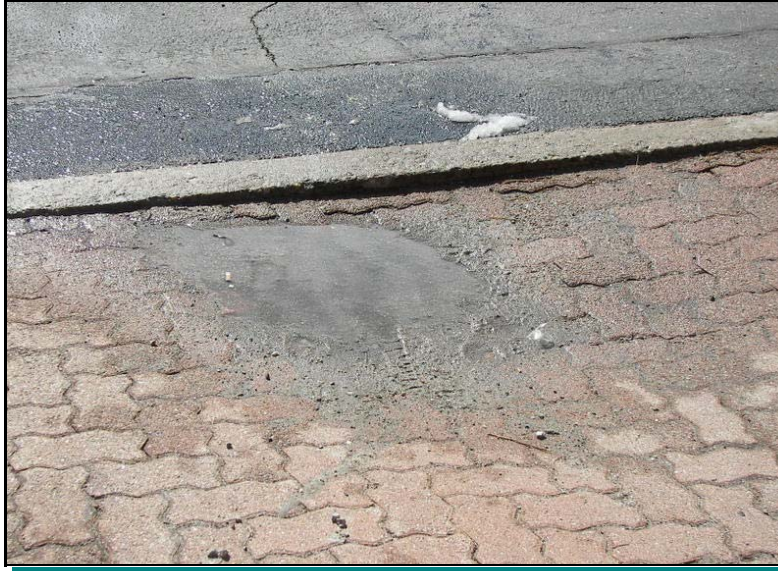
Standing water and settled brick pavers at parking area
