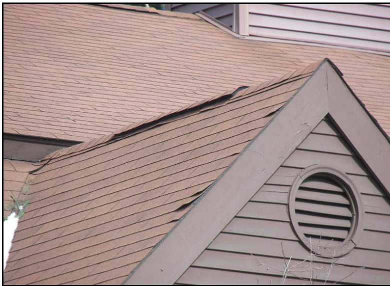
Shingle lift evident at roof
