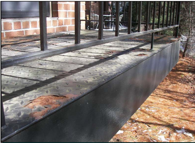
Rust, pitting and paint deterioration evident at metal balcony assembly
