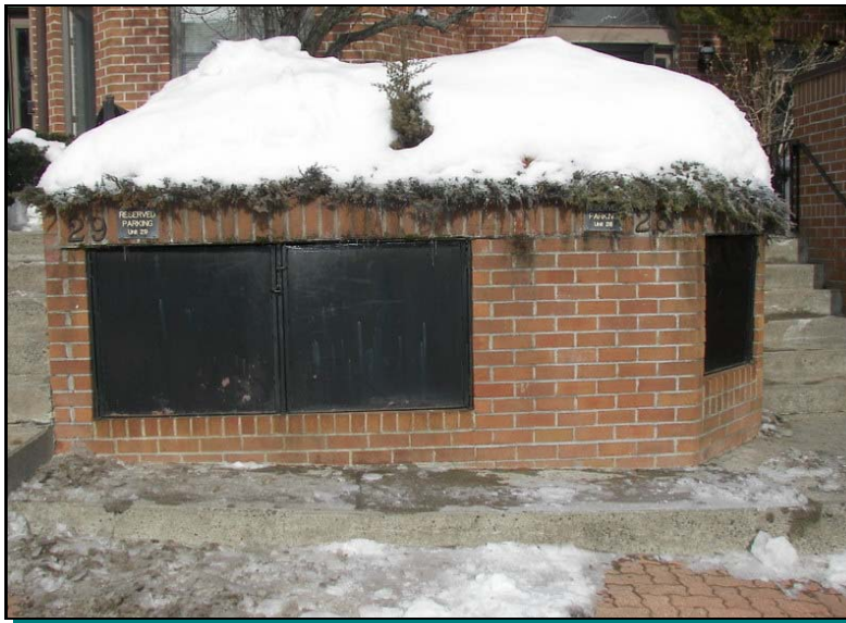
Typical brick masonry trash bins (note Homeowners are responsible for metal doors)
