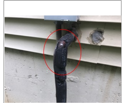
Damage / missing refrigerant line insulation.
