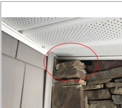
An opening above the veneer stone should be sealed as necessary.
