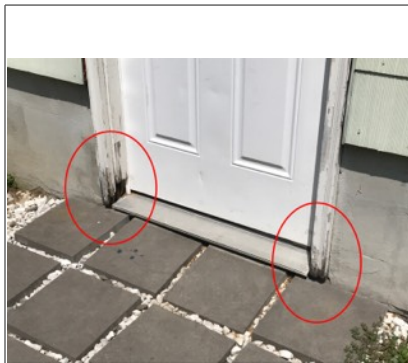
Localized rot on wood trim.
