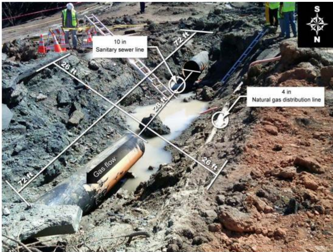
Picture of crater and ruptured pipeline.
