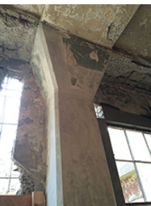
Figure 4: Powerhouse completed interior column after pumping (areas in green are historic concrete left intact)
