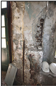
Figure 2: Powerhouse interior column deterioration
