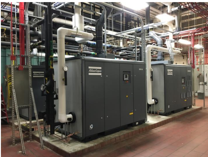
New Compressed Air System
