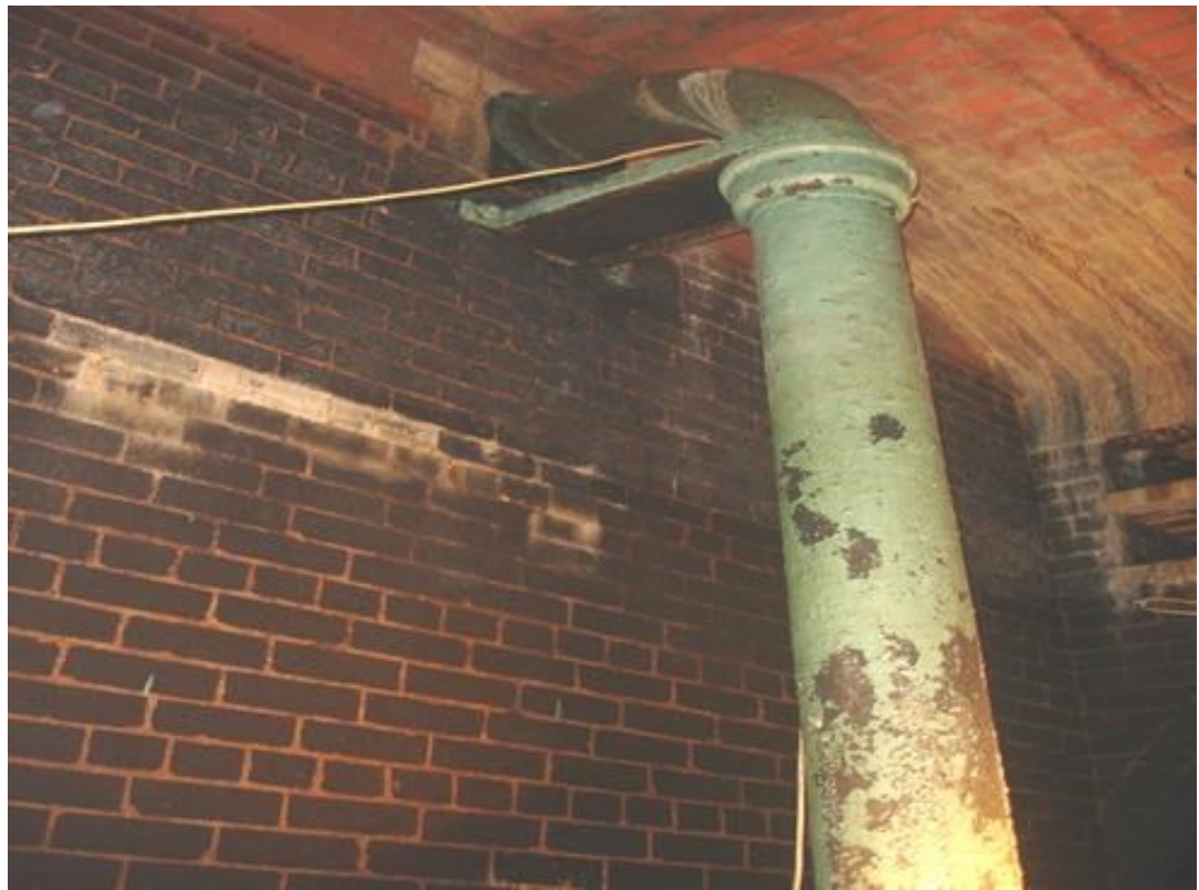
The inlet and outlet valves from the pumps and then out to the houses of Leyland.
