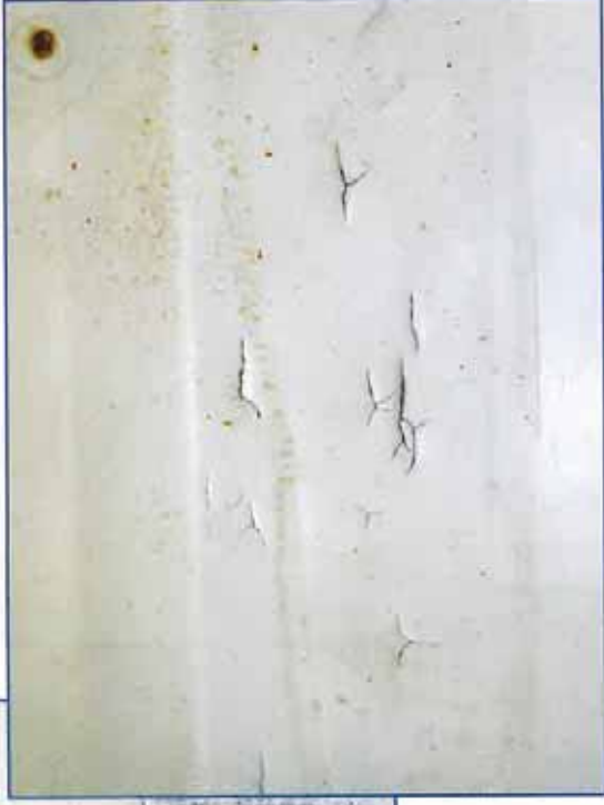
Photo 33 – View of damage on bottom of membrane.
