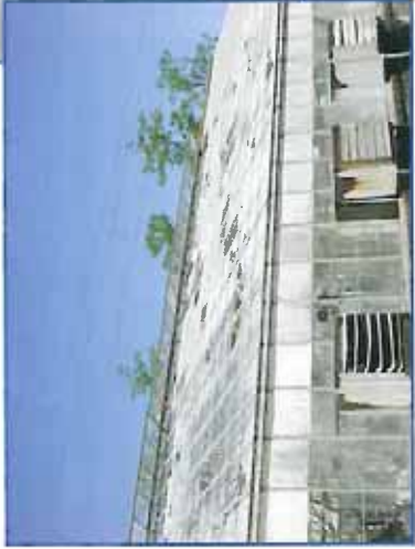
Photo 21 – Significant damage to glass panels.
