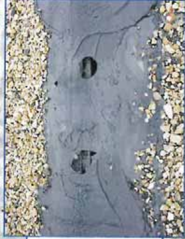
Photo 9 – Punctures in weathered expansion joint.
