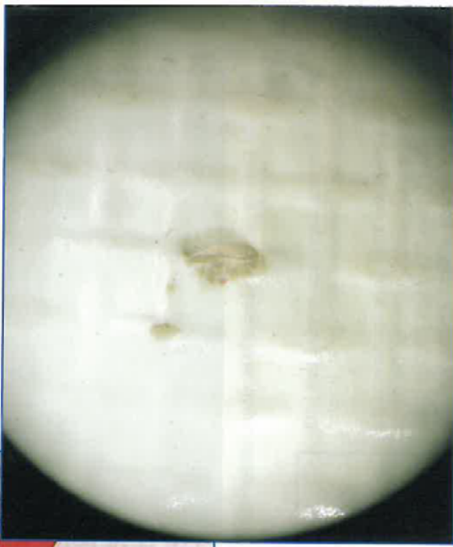
Photo 42 – Close-up view (10x) of underside of membrane showing sealant permeating the fracture. (5)
