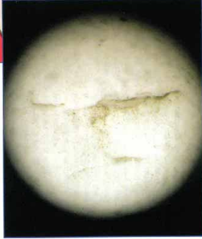
Photo 40 – Magnified view (10x) of top side of depression showing minor crack in membrane coating. (5)
