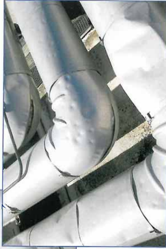
Photo 19: Dents in metal jacket on insulated piping.
