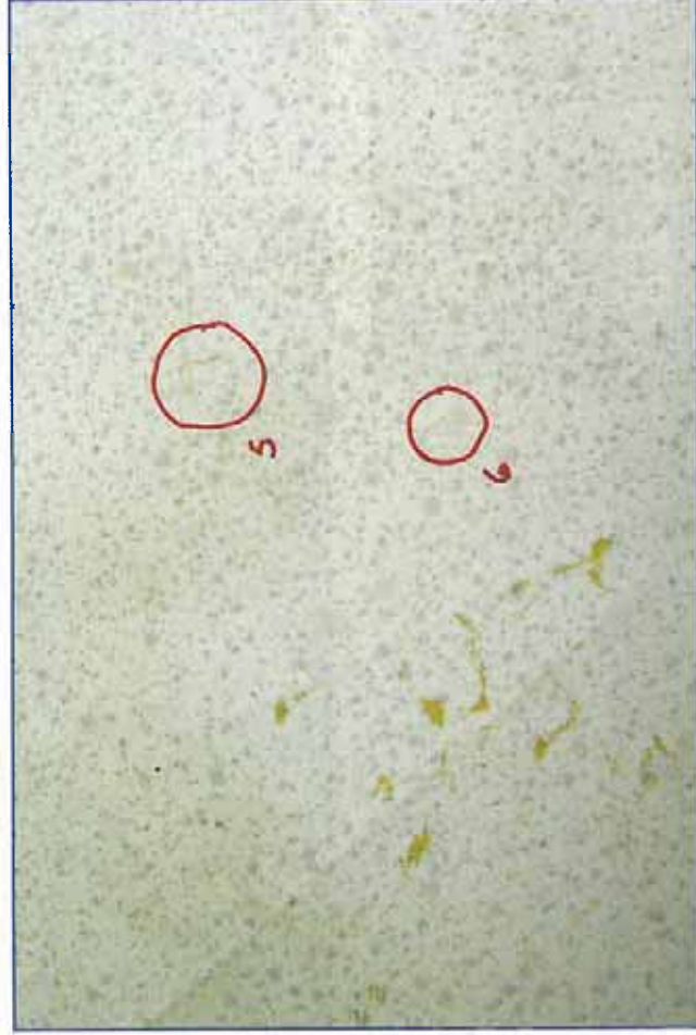
Photo 27 - Close-up view of typical damage on top side.
