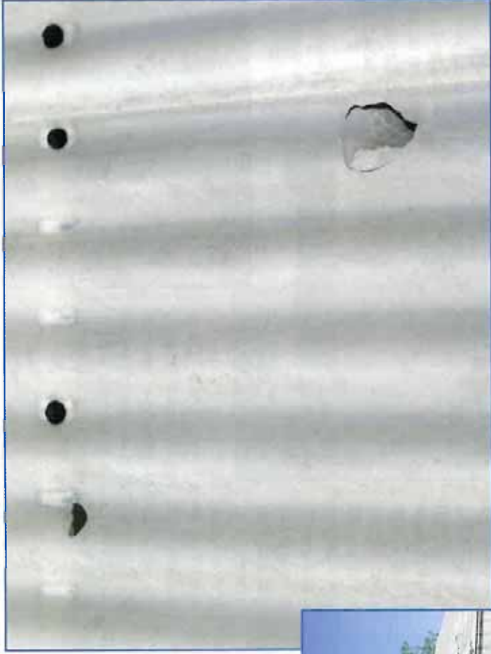
Photo 20 – Puncture in corrugated fiberglass panel.
