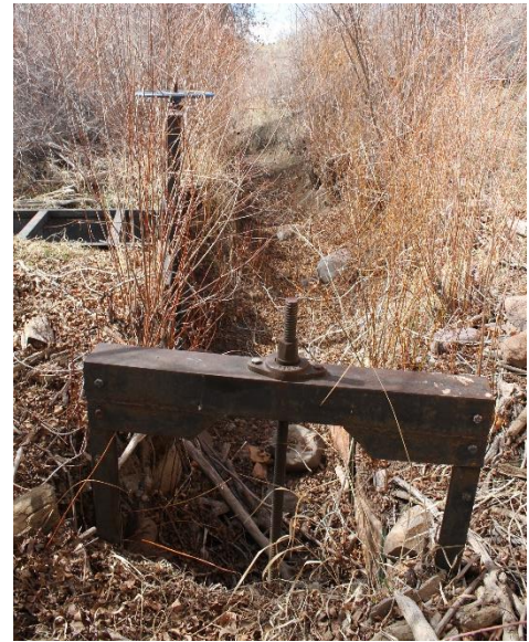
Headgate and sluice gate
