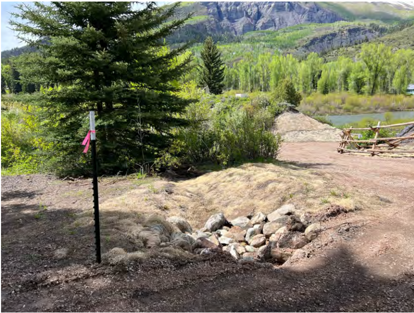
Photopoint 6. Looking north-by-northwest at a restored drainage pattern and culvert crossing on the access road upgradient of the slag pile (6/4/23).
