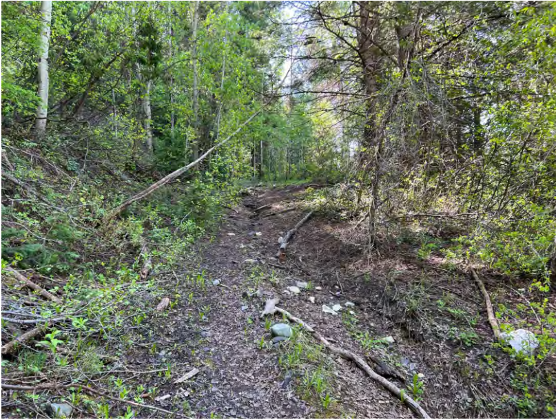
Photopoint 33. Looking west-by-northwest along the improved road (note erosion damage) off the main access road to the south boundary (6/4/23).
