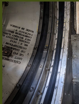
Bellmouth Seals Splice Area
