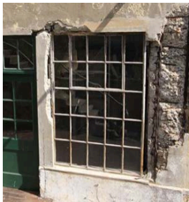
Historic window/deteriorated concrete
