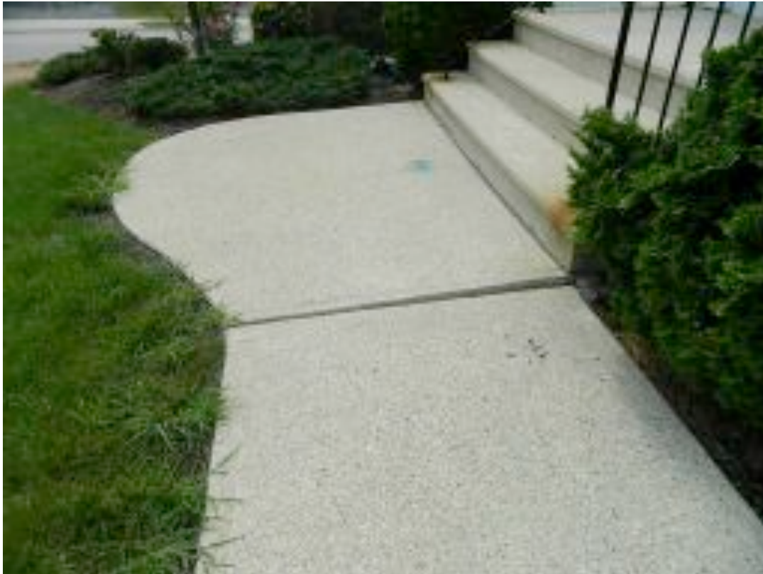
A FEW TRIPPING HAZARDS WERE NOTED (NOT WIDESPREAD)
