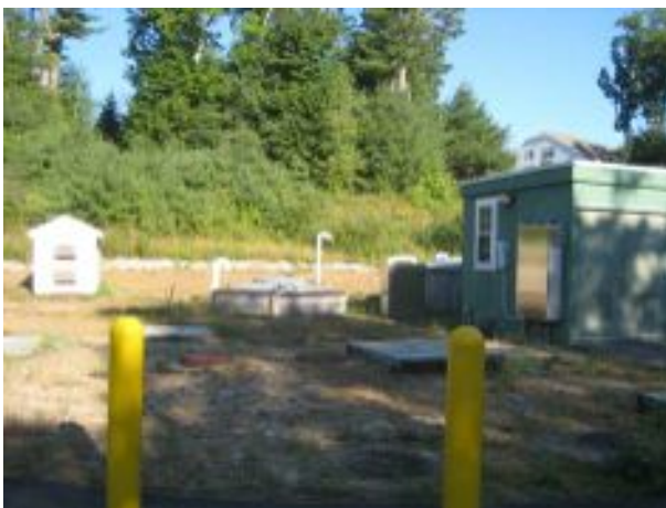
Bioclere units and Control building
