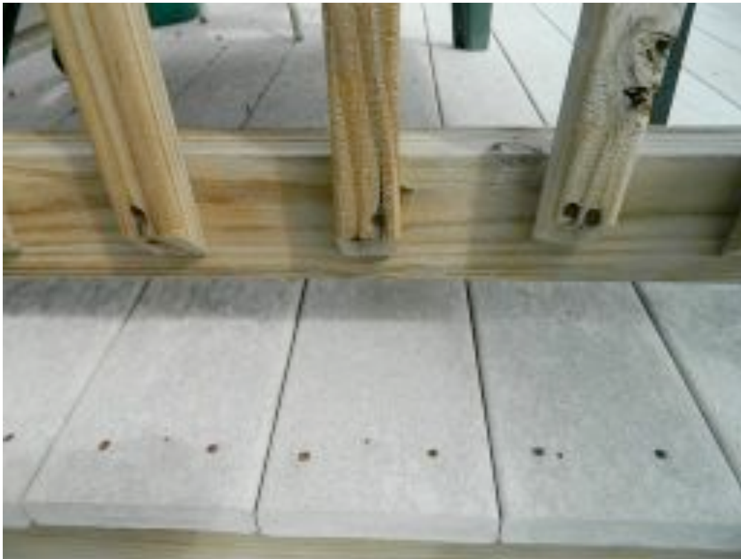
THE SYNTHETIC DECKING IS ATTACHED WITH SCREWS THAT HAVE RUSTED
