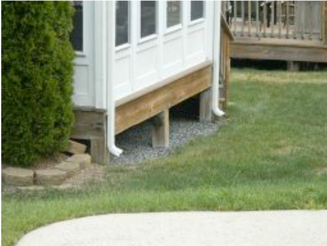
THE REAR GUTTERS SPILL TO GRADE
