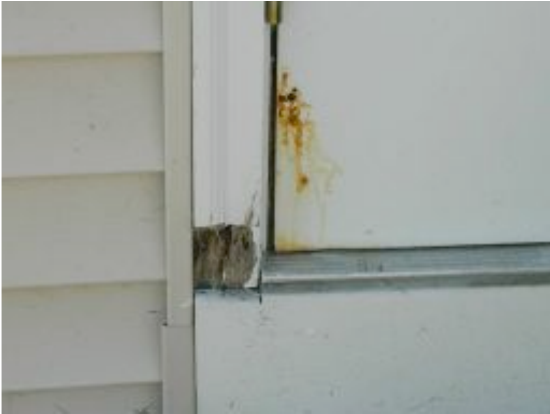
SOME SIDE UTILITY DOORS ARE RUSTING, AND SUFFERING FROM TRIM ROT
