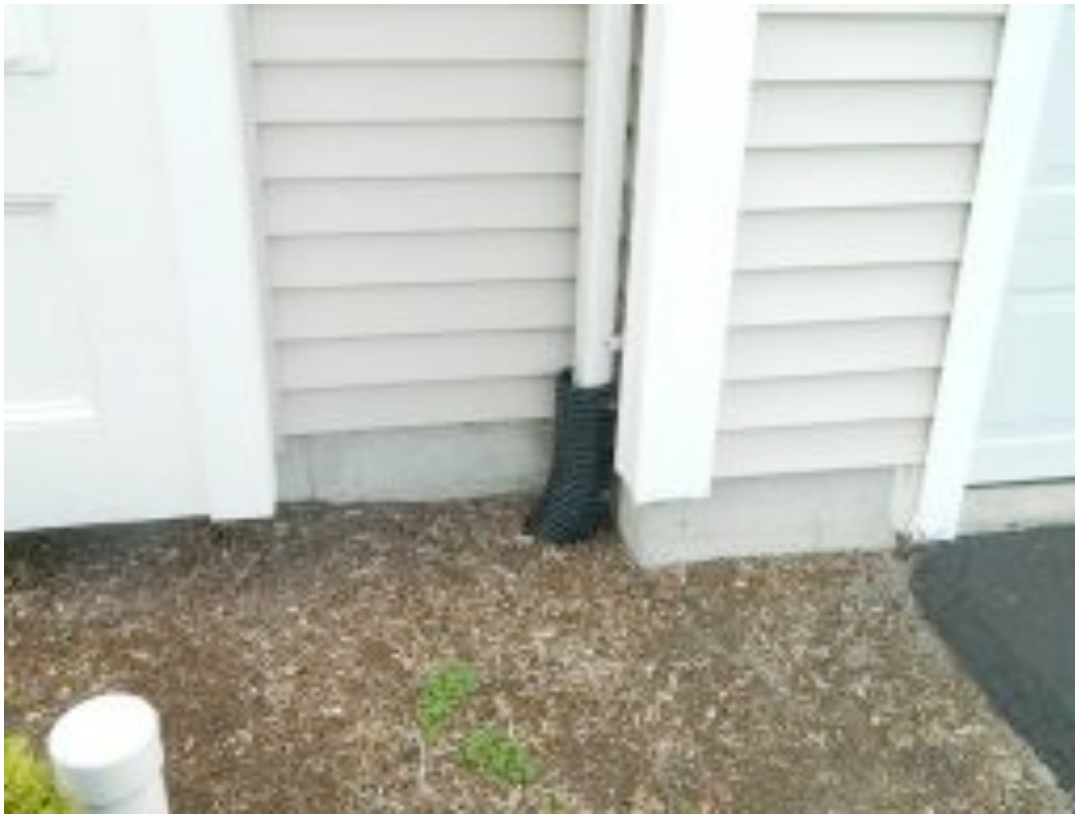
THE FRONT GUTTERS ARE PIPED TO THE SUB-GRADE SYSTEM
