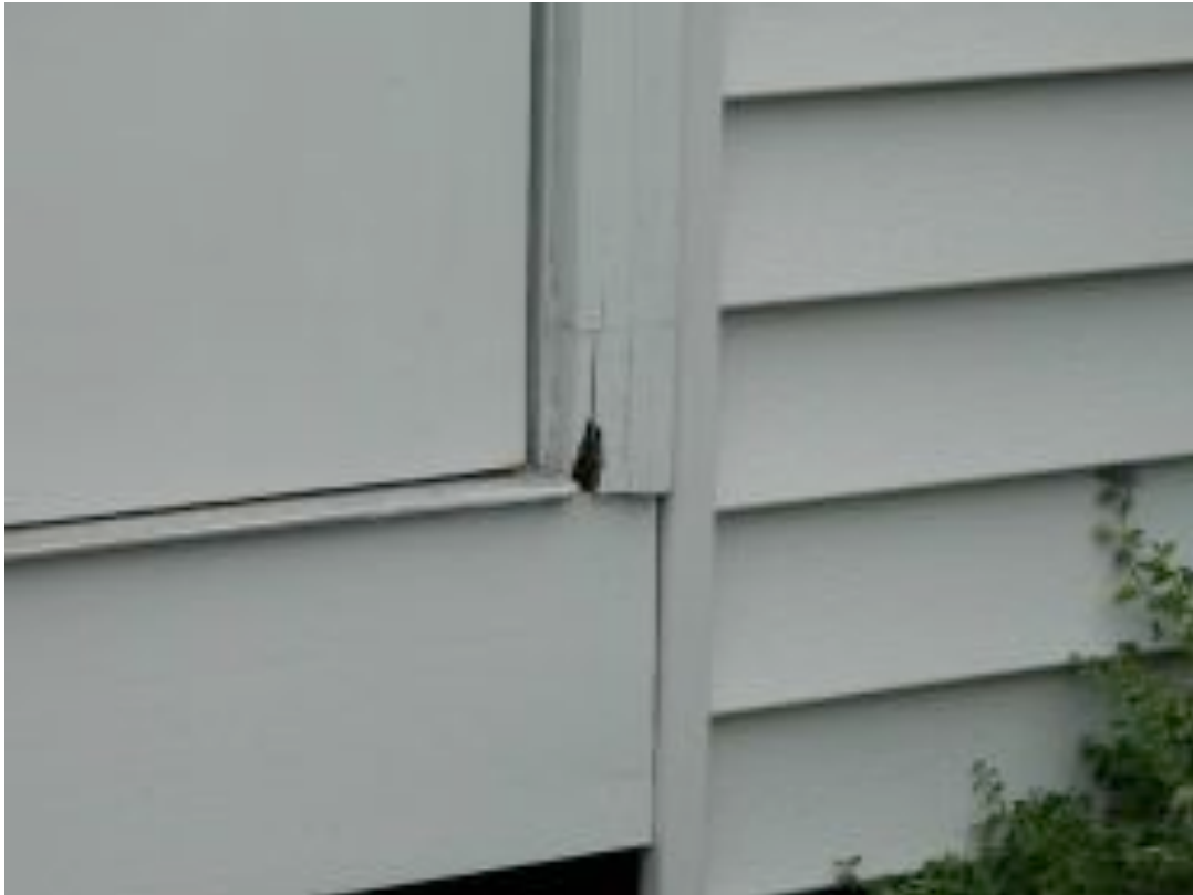
FURTHER EXAMPLE OF TRIM ROT ON A UTILITY ROOM DOOR
