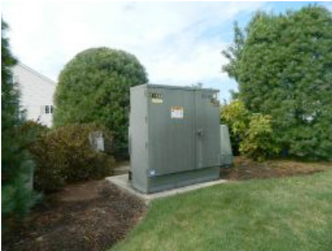
TYPICAL ON-SITE TRANSFORMER
