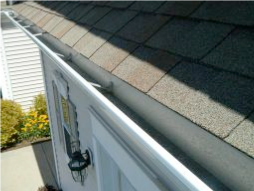
THE GUTTERS ARE ATTACHED WITH A BAR-HANGER SYSTEM (NOTE DETACHED HANGERS)
