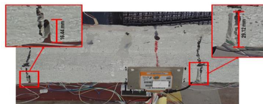
Figure 12. Example of cuts near the tendons.
