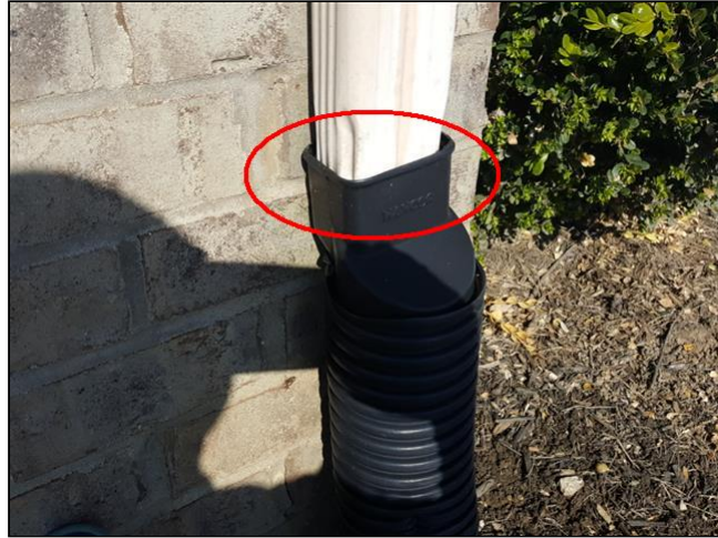
2.3 Item 8(Picture) front left corner of garage
