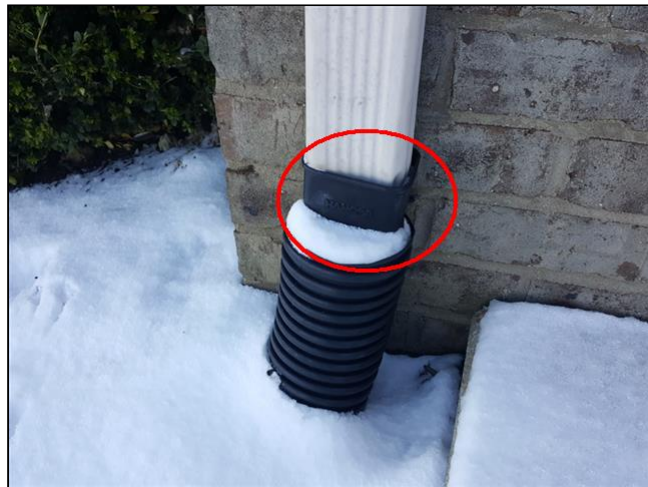
2.3 Item 10(Picture) front left corner of garage
