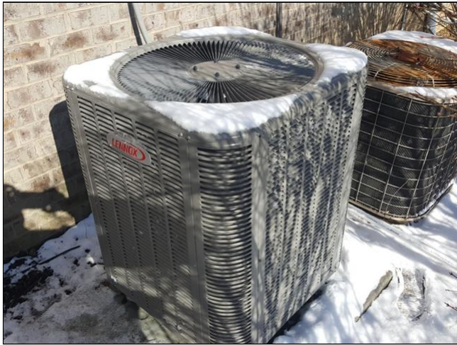
heat pump/left side of home
