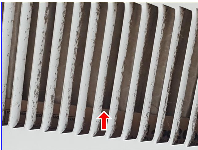
10.1.B Item 3(Picture) hallway ceiling upstairs
