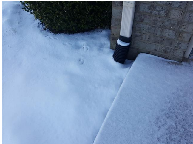
2.3 Item 6(Picture) front left corner of garage
