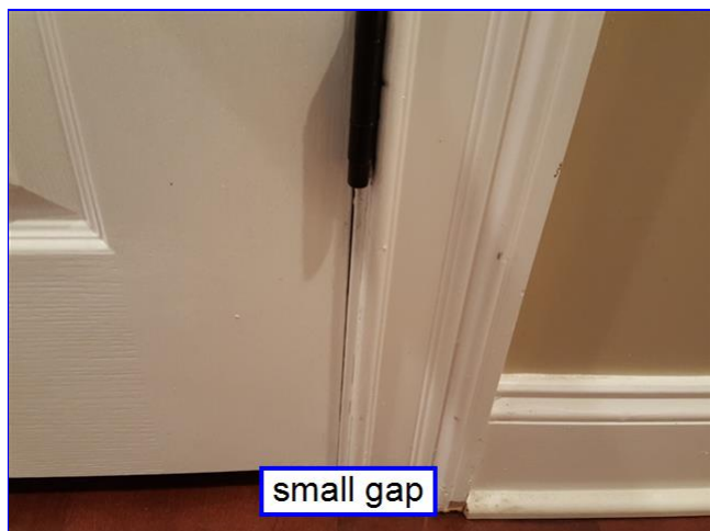
6.4 Item 3(Picture) hallway closet
