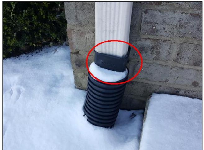
2.3 Item 10(Picture) front left corner of garage
