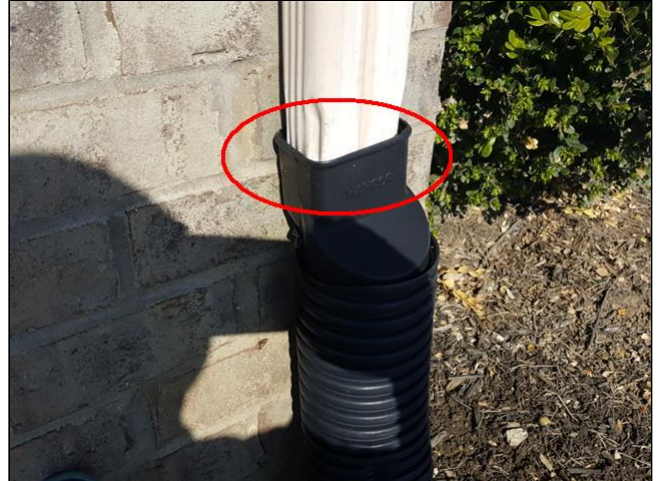
2.3 Item 8(Picture) front left corner of garage
