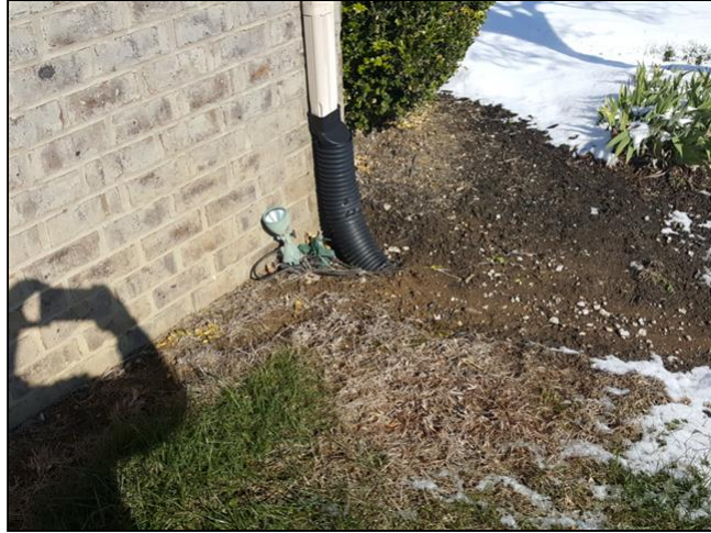
2.3 Item 4(Picture) front left corner of garage
