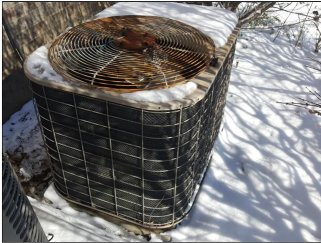
heat pump/left side of home
