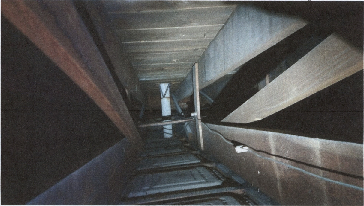
200 N. Lincoln Street – View of the 2 x 12 rafters and the diagonal bracing closer to the middle of the building.
