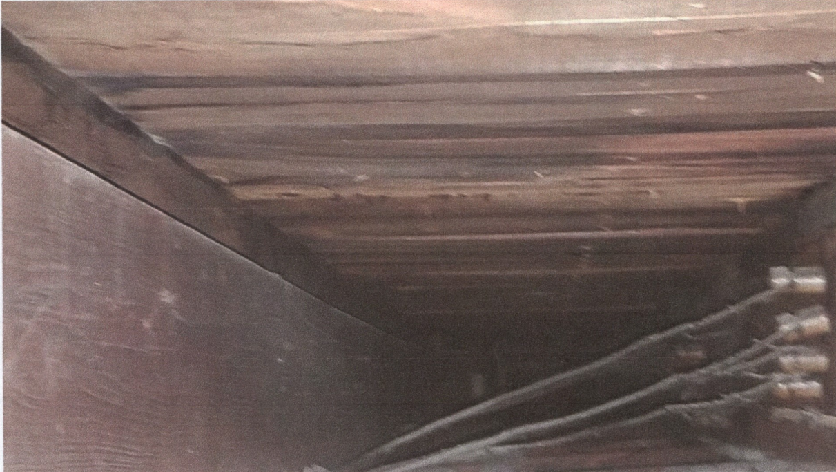
200 N. Lincoln Street – View of the 2 x 12 rafters and the sistered rafter and roof decking.
