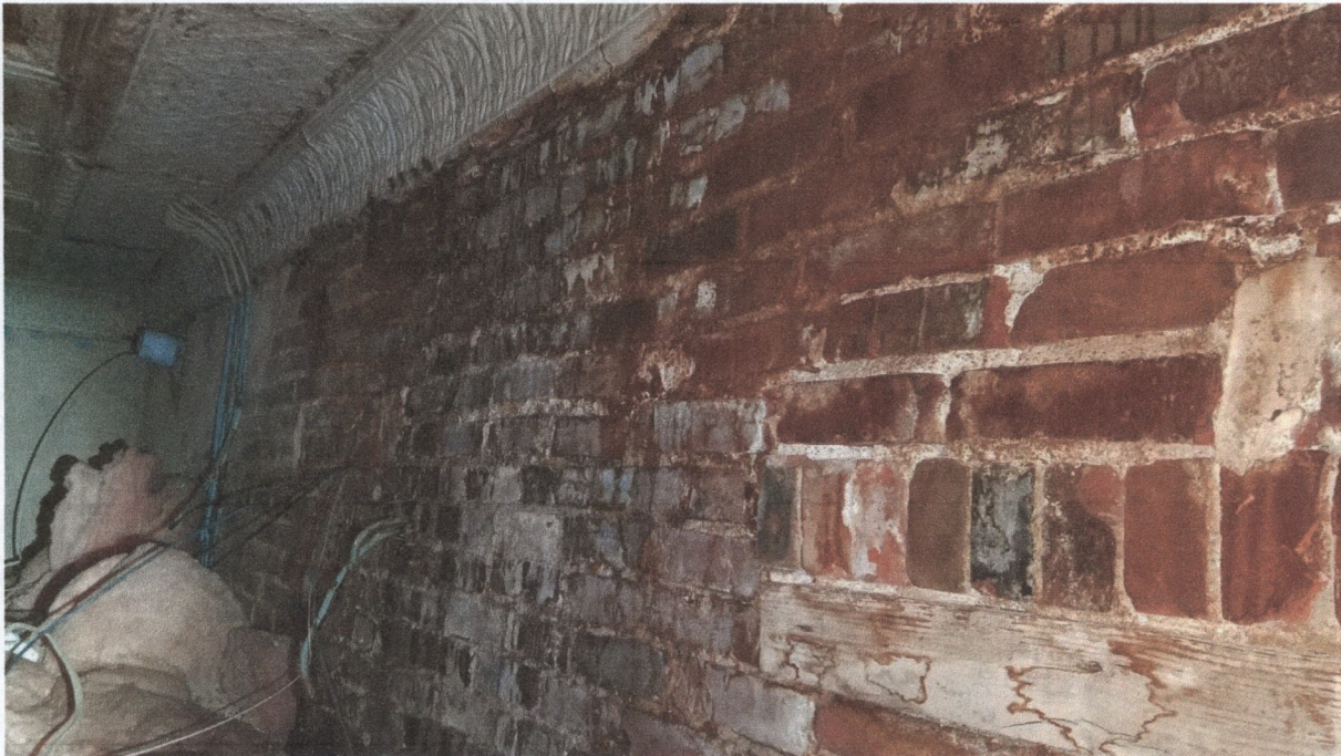
200 N. Lincoln Street – View of the interior side of the rear wall of the building showing the water damage to the brick masonry.
