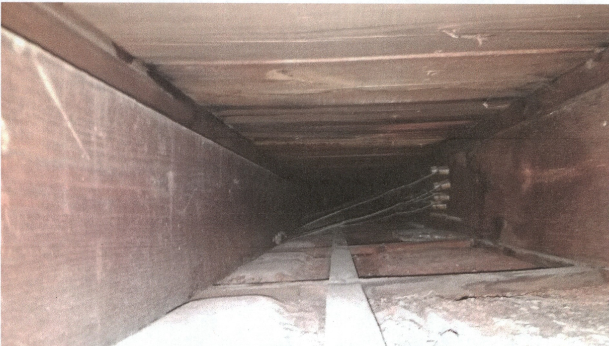
200 N. Lincoln Street – View of the roof decking and the rafters near the rear wall of the building facing the north.
