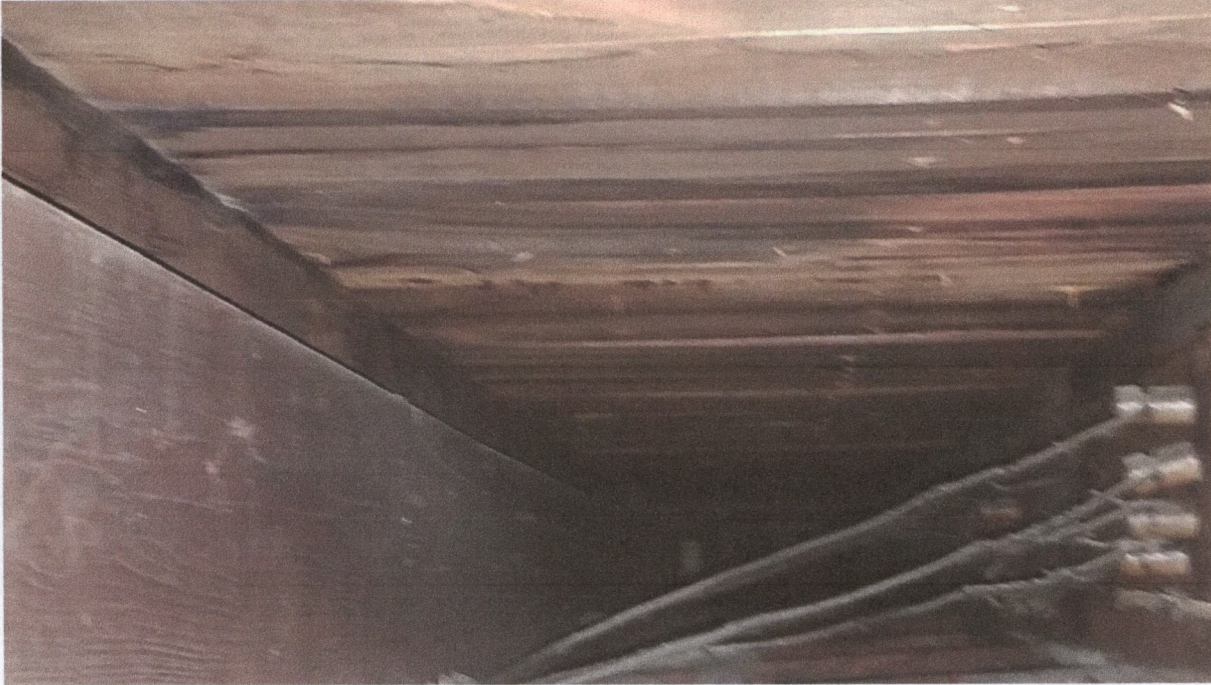
200 N. Lincoln Street – View of the roof decking and the rafters near the rear wall of the building facing the north.
