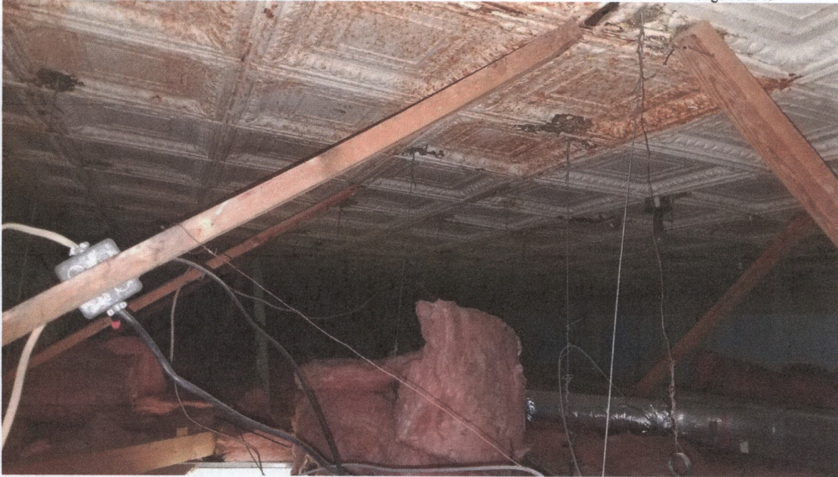
200 N. Lincoln Street – View of the original ceiling showing the rusting and damaged ceiling tiles.
