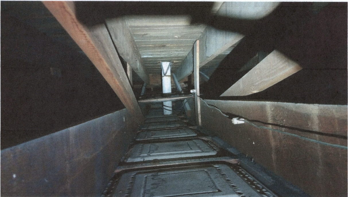
200 N. Lincoln Street – View of the 2 x 12 rafters and the diagonal bracing closer to the middle of the building.
