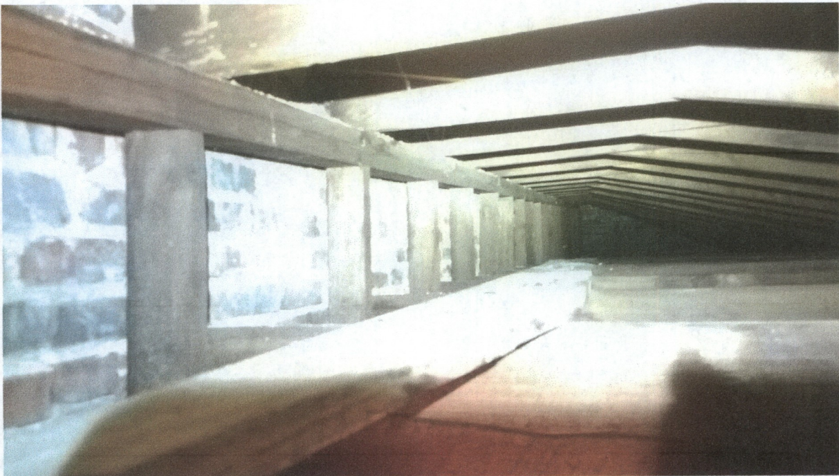
200 N. Lincoln Street – View of the south wall of the building showing the stud knee wall and the 2 x 12 rafters.
