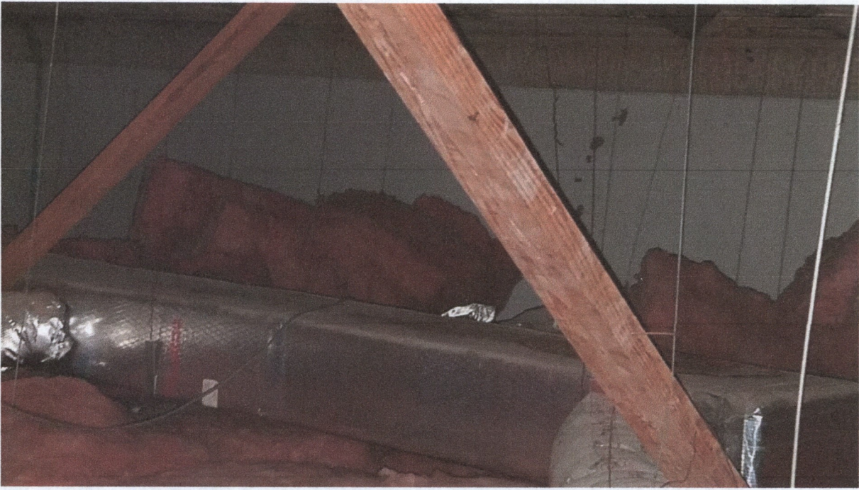
200 N. Lincoln Street – View of the original ceiling and the space above the dropped ceiling.
