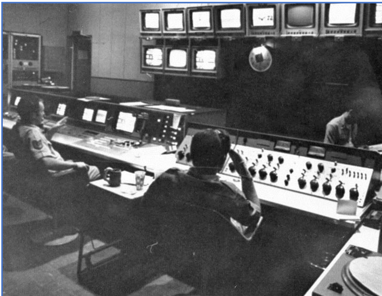
The TV Control Room.
