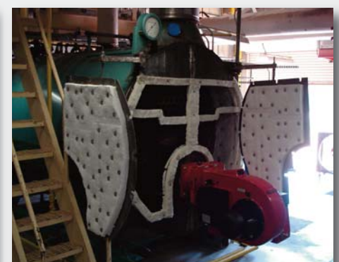
End Result. A more fuel efficient boiler with no Cleaver Brooks parts.
