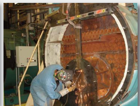
Step 2. Manufacture a new inner plate with studs to accept the new door.
