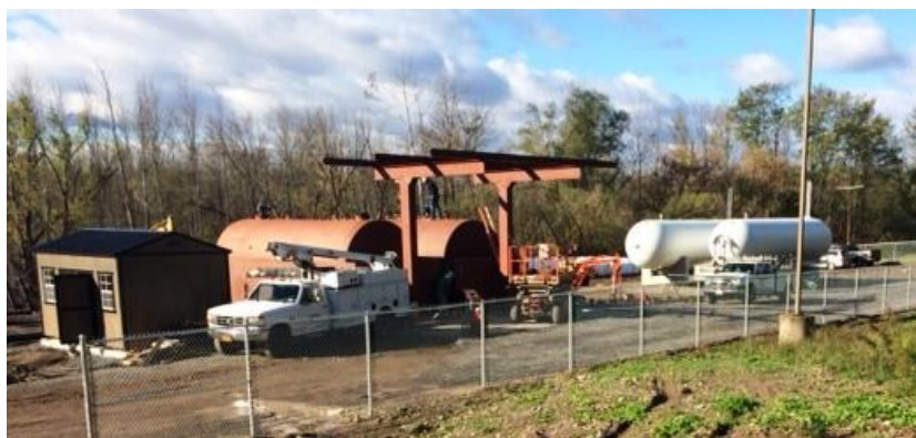
New Bulk Plant storage facility in progress located on Bloom Road, Newark.
