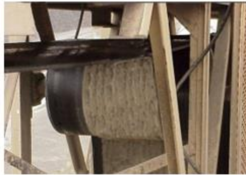
This photo shows buildup on a bend pulley. In 2024 a miner lost a thumb when he removed a guard and began to clean a rotating bend pulley with a 15-inch-long pry bar.
