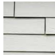
Gaps in Fiber Cement
