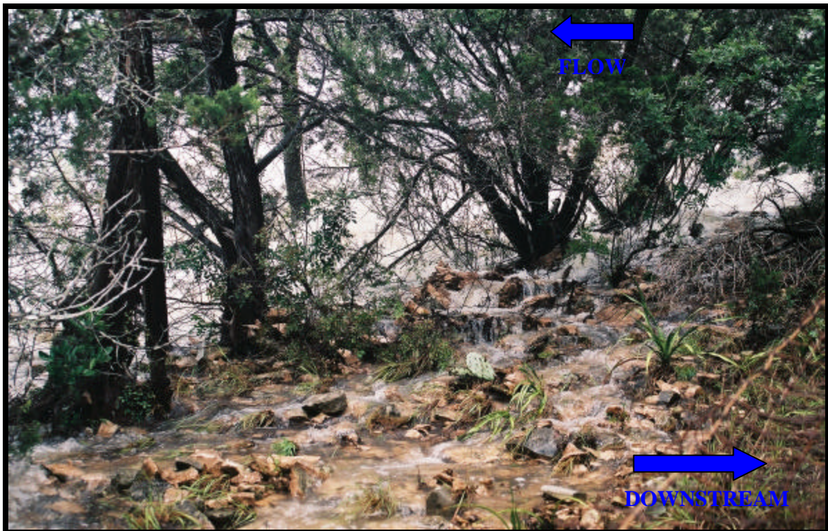
Photo 15 View of overtopping and erosion of left overbank, looking left. (Friday, July 5 th )
