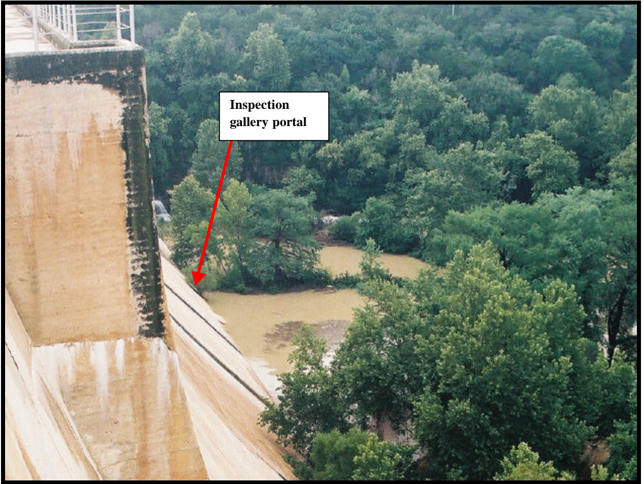
Photo 24 View of concrete gravity section-river, looking left and downstream. Note the tailwater level is just below the inspection gallery portal. (Saturday, July 6 th )
