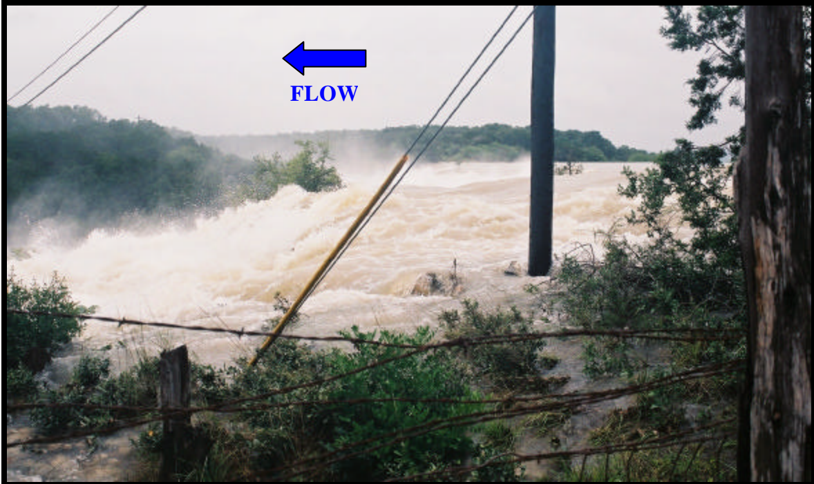
Photo 17 View of discharge over emergency spillway, looking upstream from the left overbank. Note the overtopping of the left overbank in the foreground. (Friday, July 5 th )
