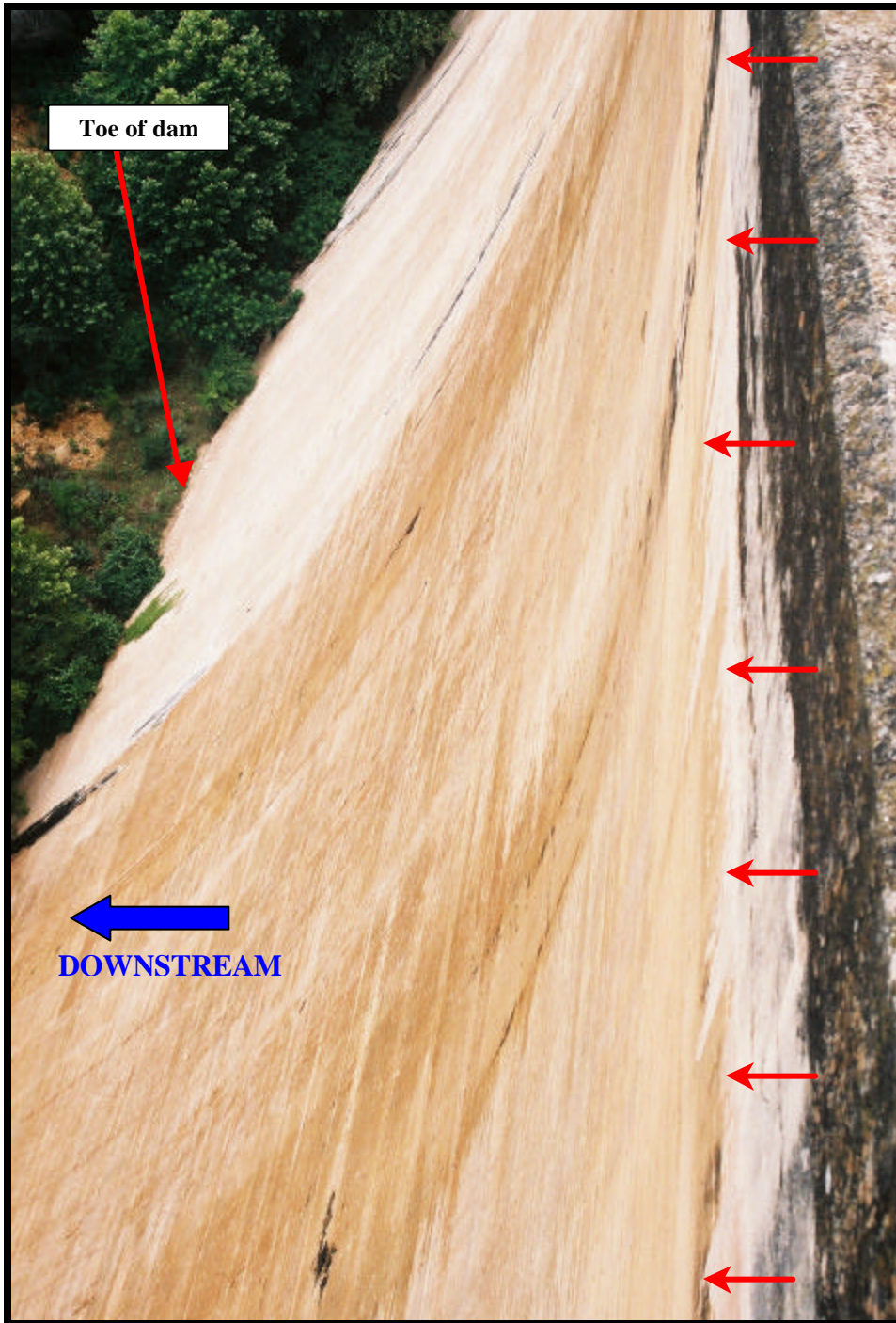
Photo 23 View of concrete gravity section-river, looking right. Note the dampened section along a horizontal line. (Saturday, July 6 th )
