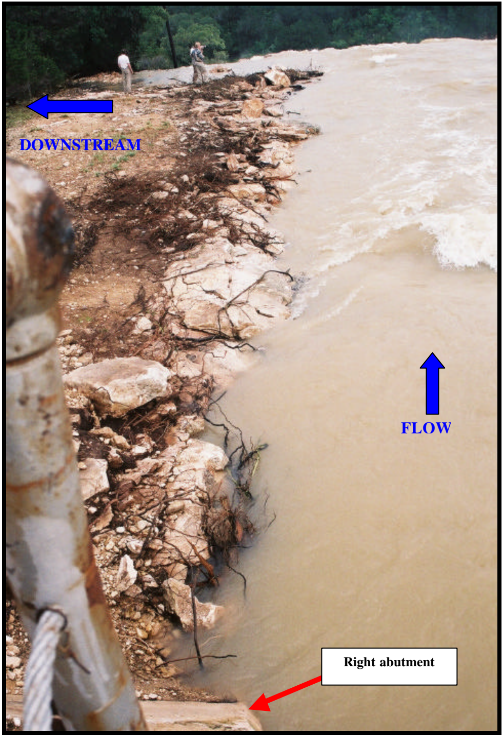
Photo 27 View of erosion along right abutment, looking right. (Saturday, July 6 th )
