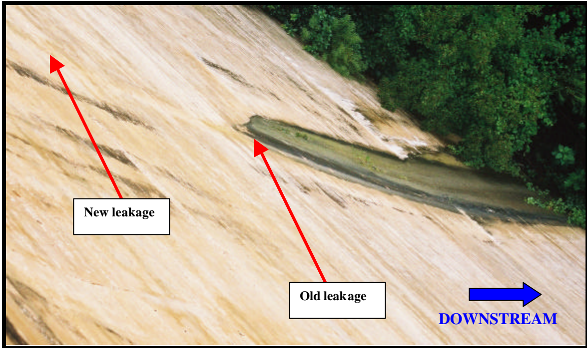
Photo 3 View of vertical crack in concrete gravity section-left abutment, looking right and downstream. Note the new leakage through the crack versus older, algae-stained leakage areas. (Friday, July 5 th )
