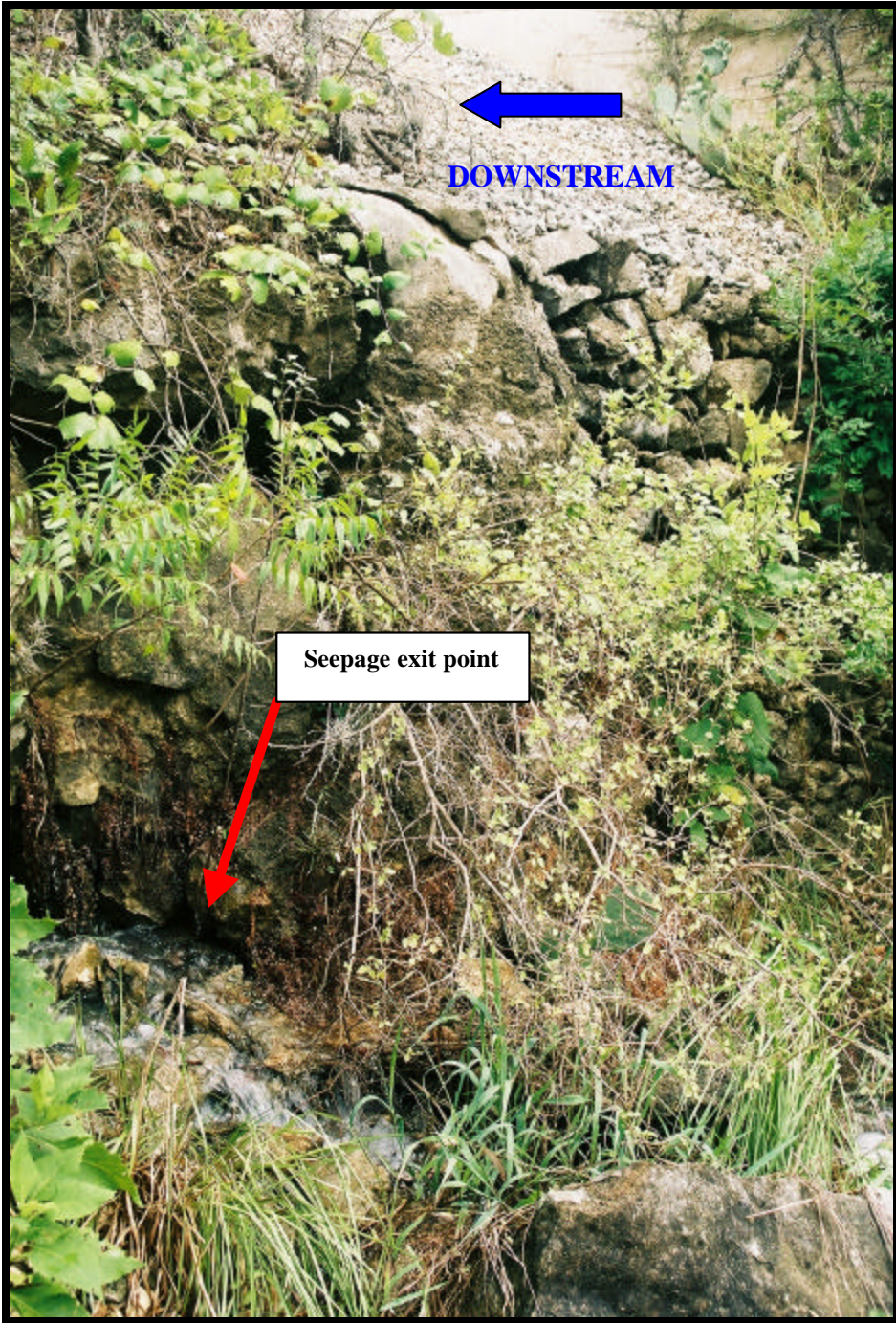
Photo 25 View of foundation seepage downstream of toe of dam, looking right. (Saturday, July 6 th )
