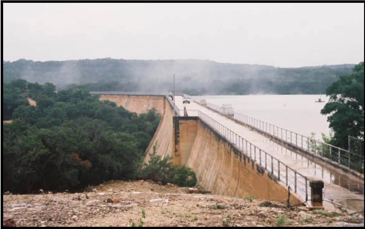
Photo 1 View of left abutment and crest of concrete gravity section, looking right. (Friday, July 5 th )
