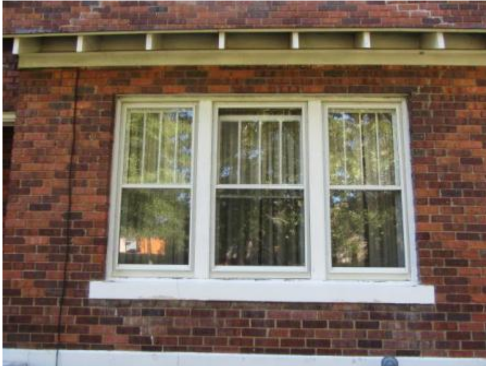
Figure 58. NCDOT Survey #15, Edwards House (GF-8177), 7210 Burlington Road, Guilford County, detail of typical tripartite window, west window bay, looking east.
