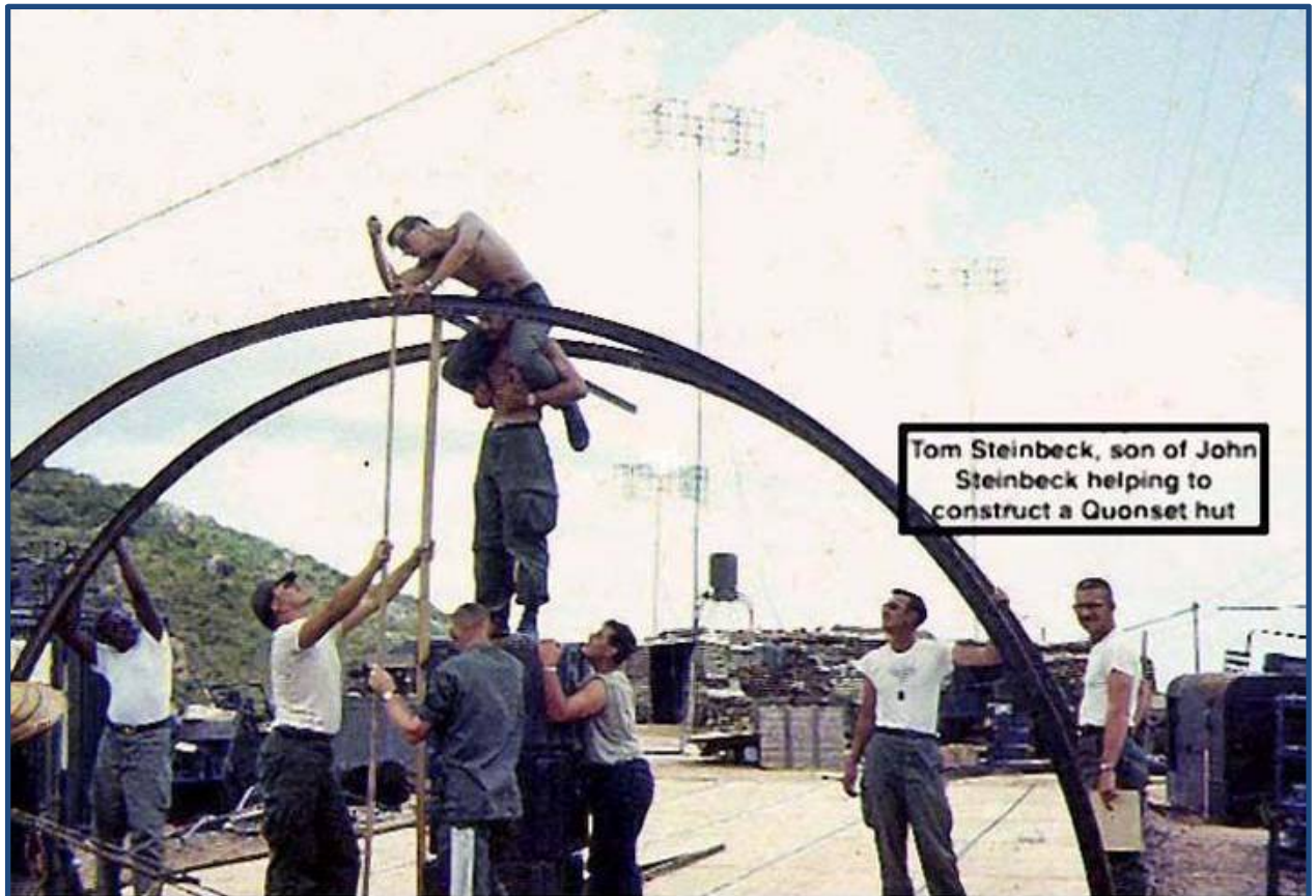
Tom Stienbeck, son of the author, John Steinbeck, helping to construct a Quonset Hut.
