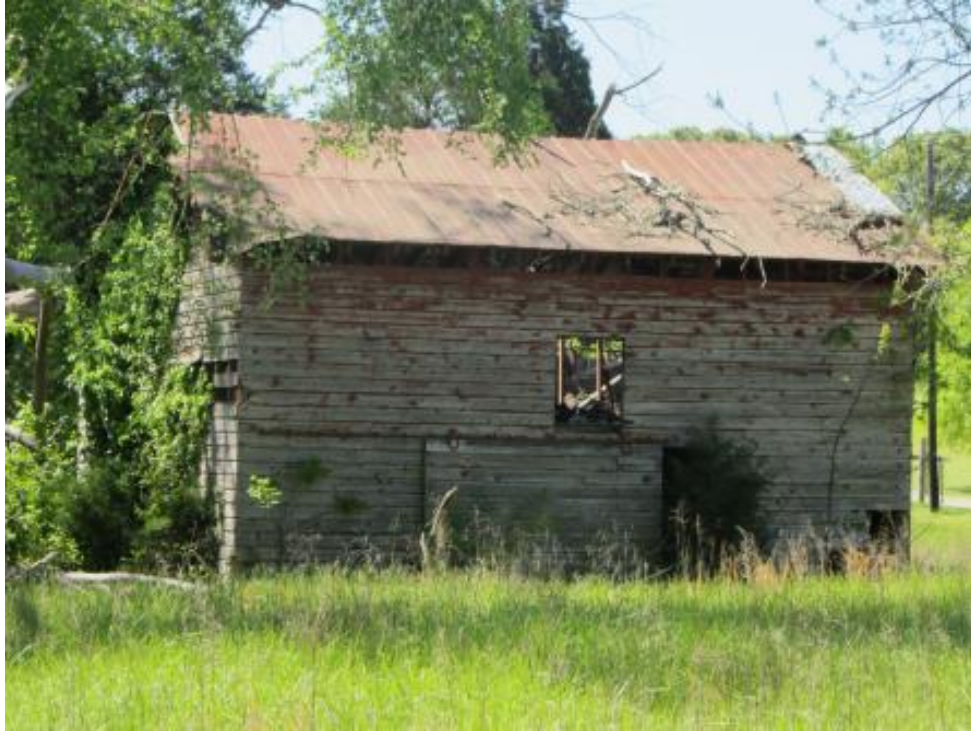
Figure 86. NCDOT Survey #12, Ingle House (GF-8174), 7232 Burlington Road, Guilford County, view of derelict barn that still stood on property when photographed in April 2012, but had been demolished by September 2012.
