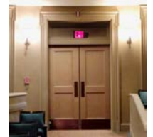
Before (top): cracks at door surround; After (bottom)
