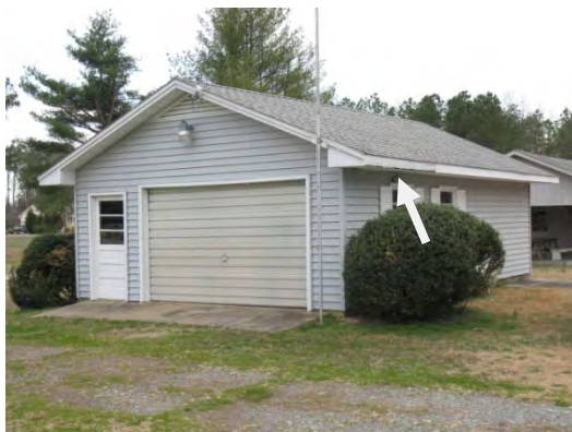
Photo 37 - Storage shed roof and siding in good condition - eave trim cover damaged
