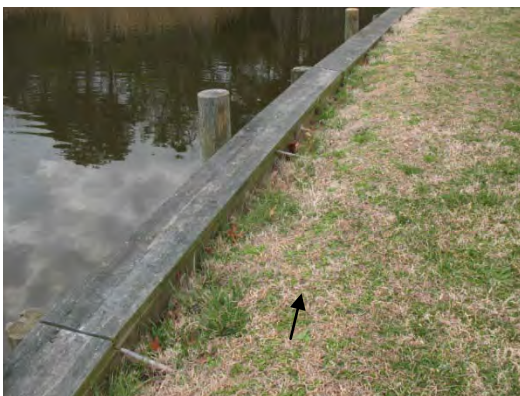
Photo 70 - Erosion is occurring behind the bulkhead near the parking area
