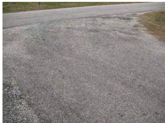
Photo 4 - Landsend East at intersection with Corrotoman Dr. is deteriorating and requires patching
