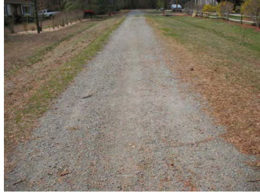
Photo 10 - Middle Rd. with loss of gravel along edges and vegetation encroachment
