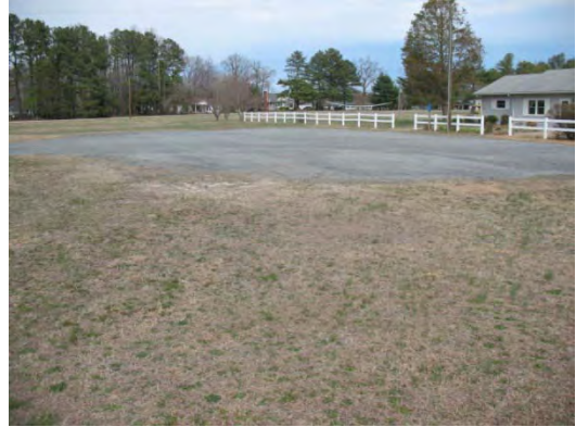
Photo 6 - Clubhouse asphalt parking area requires edge patching and vegetation removal
