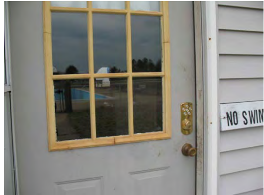
Photo 22 - Rear door glazing frame is cracked
