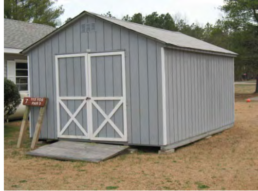
Photo 40 - Garden shed is in fair condition and needs to be reset on foundation blocks
