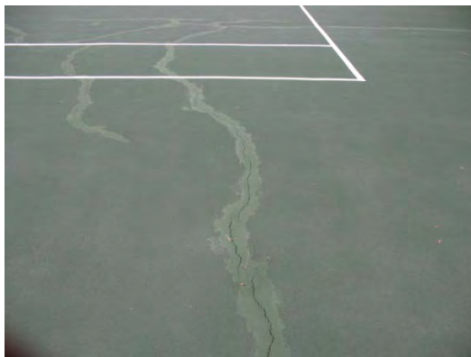
Photo 55 - Repaired crack that has re-opened
