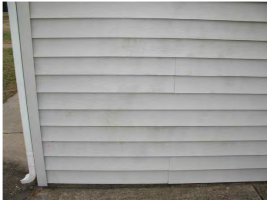
Photo 19 - Typical vinyl siding - dark spots are dirt stains that can be cleaned
