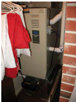
Photo 35 - Clubhouse gas furnace
