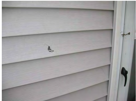
Photo 20 - One area of cracked siding was observed - located near men's room door
