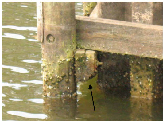
Photo 69 - Bottom frame timber is rotting
