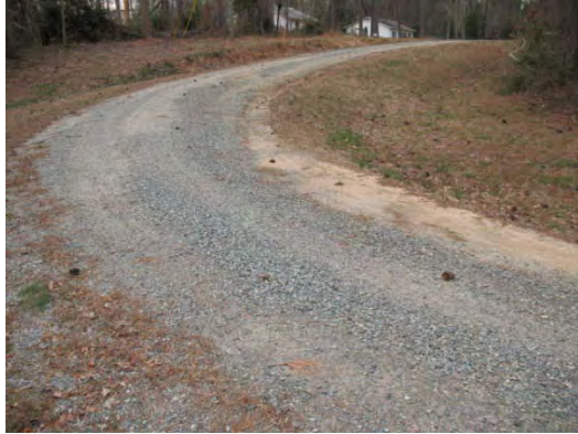
Photo 9 - Meadowview Ln. with erosion along edge
