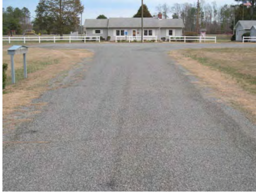
Photo 5 - Asphalt pavement at drive to clubhouse with edge cracking - vegetation in pavement will shorten life
