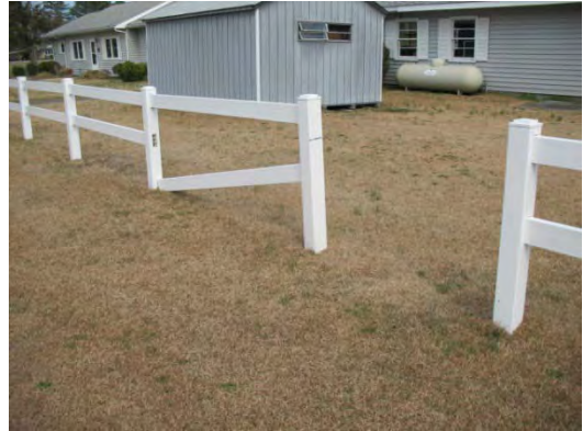
Photo 16 - Vinyl fences expand and contract causing rails to come loose
