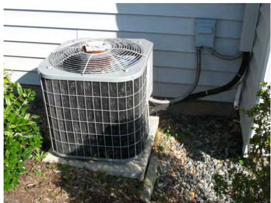
Photo 36 - Clubhouse outdoor unit for cooling
