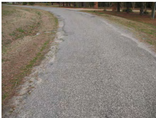
Photo 3 - Edge cracking and loss of asphalt pavement on E. Highview - requires cutting existing asphalt parallel to edge and patching
