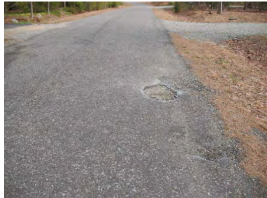
Photo 2 - Example of pothole on Corrotoman extension
