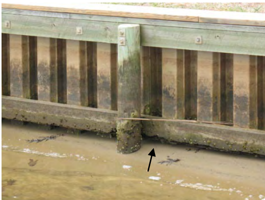
Photo 68 - Bottom frame timber is rotting
