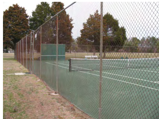
Photo 56 - Tennis court fencing has numerous areas of rust
