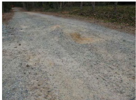
Photo 8 - Sandy Ln. with ruts and potholes
