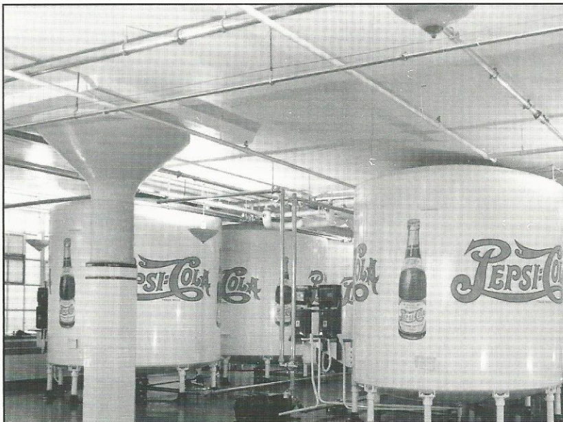
Pepsi Concentrate Storage Tanks
