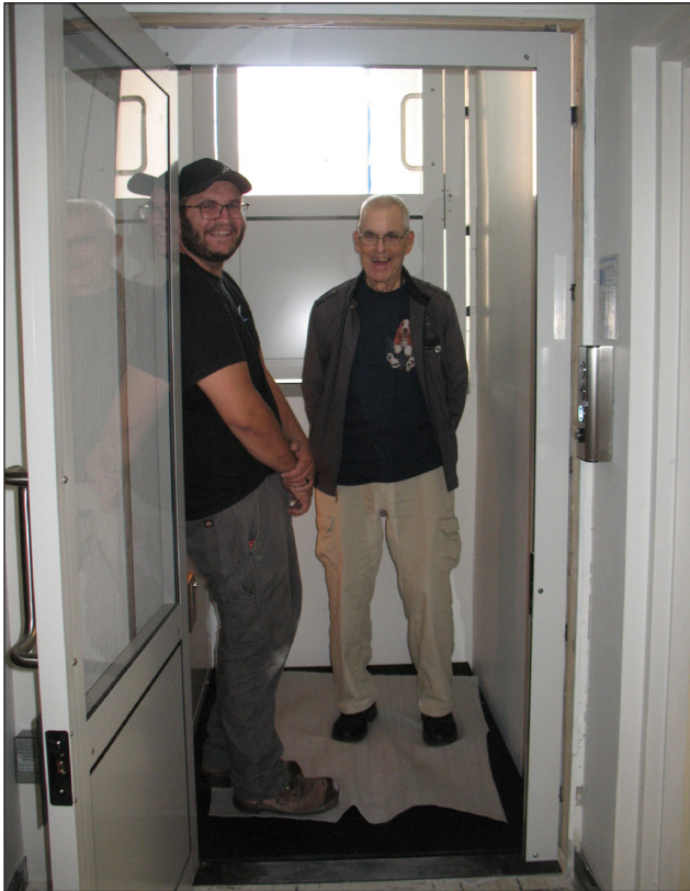
Lyle Swenson and Matt Toering, installer for Access Elevator & Lifts Inc. (AEL), are first to ride in the new chair lift at the east entrance of the CRC. The lift can go down to the basement or it can go up to the Corn Palace Room. It has room for a wheel chair, motorized or not and another person. The base is 42 x 60 inches and will hold 750 lbs. A little fine tuning and signage and the project will be finished. We are happy to be nearing the end of this project and thanks to those who helped make it a reality.
