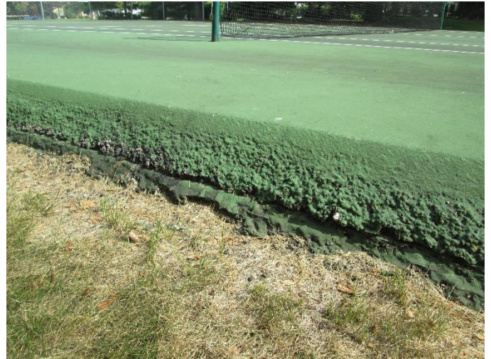
Evidence of previous tennis court overlayment
