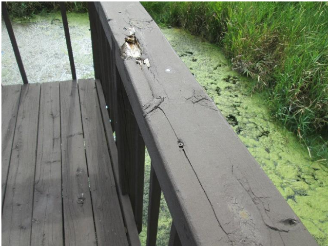
Deteriorated wood at large pier
