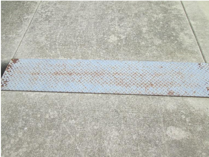
Surface rust on plate at spillway walking surface
