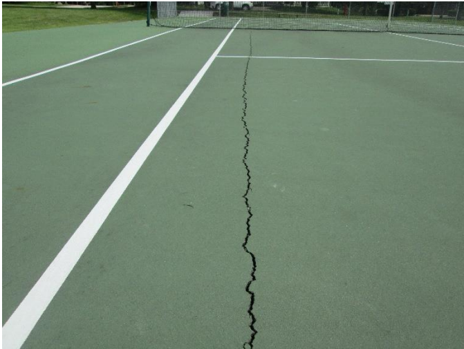
Significant surface cracking
