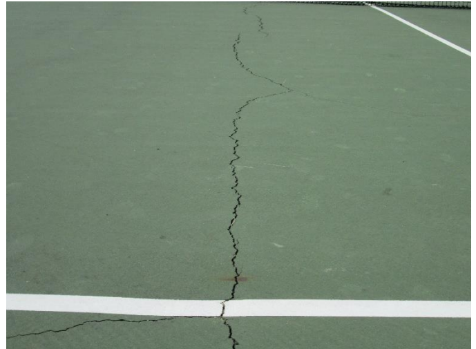
Significant surface cracking
