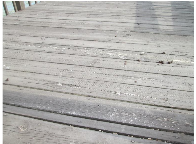
Deteriorated wood at large pier
