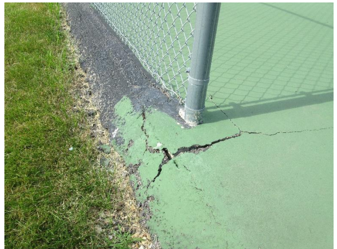
Minor heave at fencepost footing
