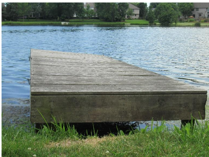
Settlement and deteriorated wood at small pier
