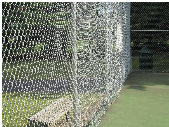
General wear noted at fencing
