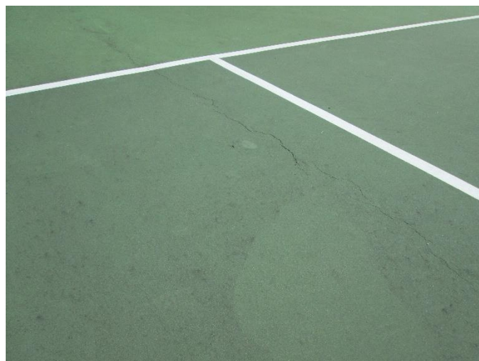
Color coat deterioration and surface cracking
