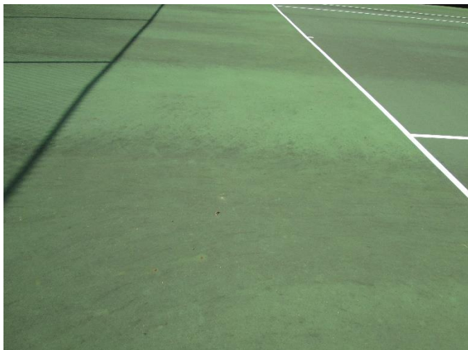
Color coat discoloration
