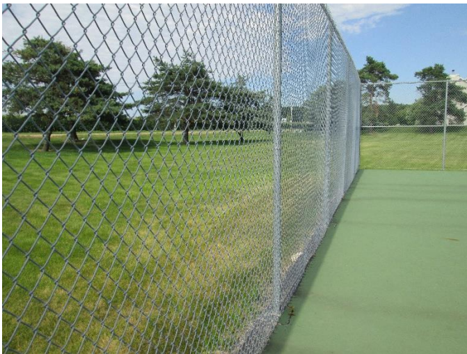
Minor general wear at fence
