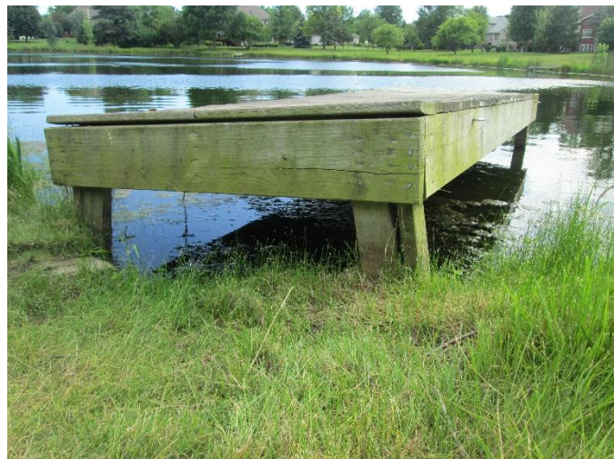
Settlement and deteriorated wood at small pier
