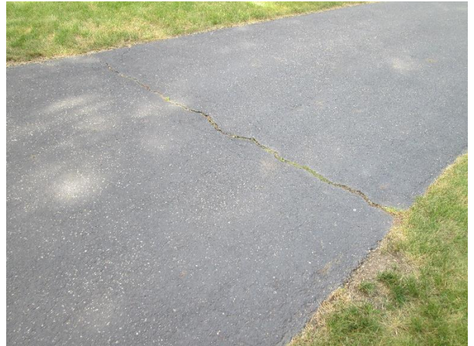
Pavement cracking and minor surface deterioration
