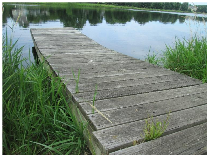
Settlement and deteriorated wood at small pier
