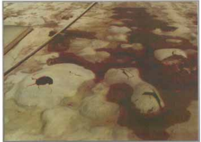
Blisters in spray-applied polyurethane foam roof system.
