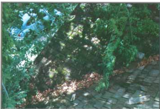
Moss growth on wood shingle roof covering.
