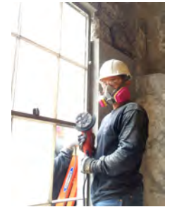
Team member grinding surface of repairs to achieve historic texture; safety first
