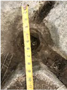
Condition assessment revealed non-functioning drainage pipe
