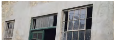
Top: Exterior front façade in progress; Bottom: Exterior front façade repairs completed, prior to painting
