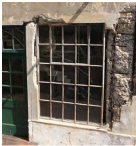
Historic window/deteriorated concrete
