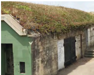
Before: Deteriorated condition, visitor safety compromised
