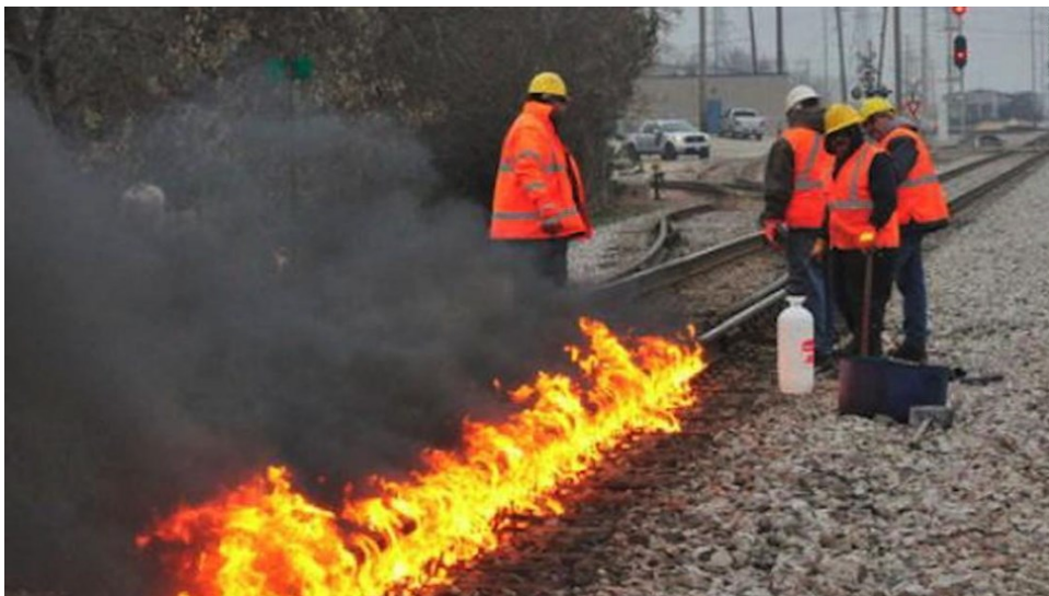
Crews using a firesnake to defrost tracks. Firesnake is chemically impregnated rope laid in ten-foot section to heat rails.
