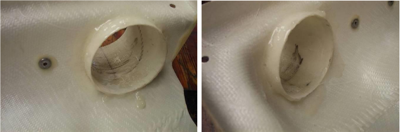
Figure 36. Air Filter Box Plumbing – Incorrect
