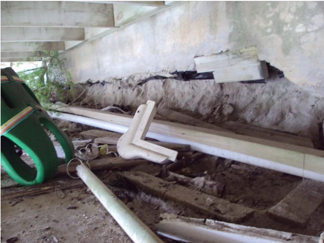
12. Lot 14, Block 3 – Foundation Failure (5 - Critical)
