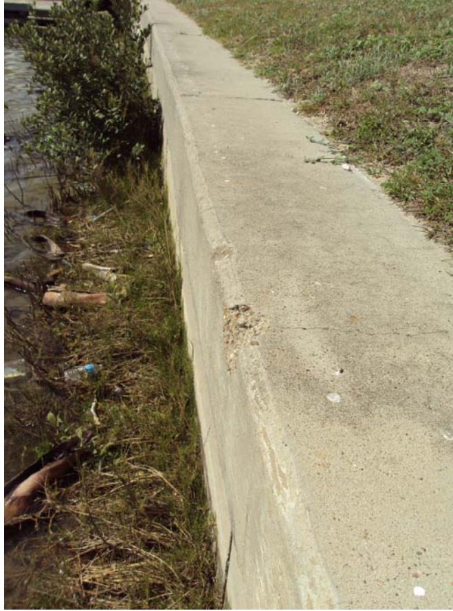
3. Lot 16, Block 3 – Minor Cap Damage (2 - Satisfactory)
