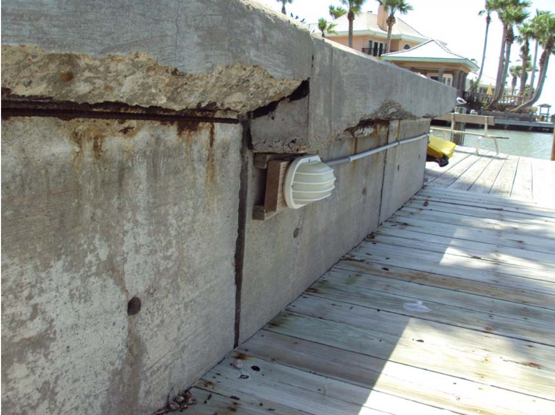
8. Lot 3, Block 3 – Major Cap Damage (4 - Poor)
