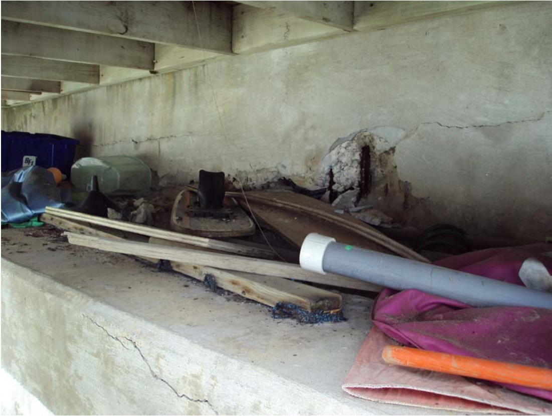
11. Lot 14, Block 3 – Foundation Failure and Moderate Cap Damage (5 - Critical)
