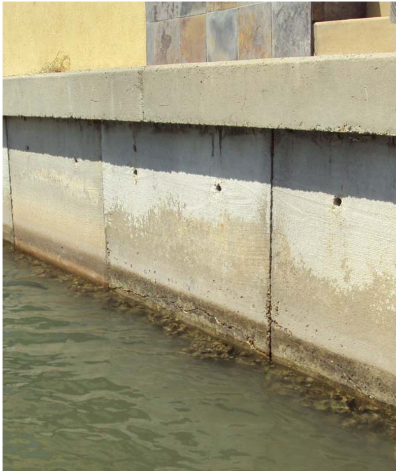
14. Lot 2, Block 2 – Cracked Bulkhead Panel (4 - Serious)
