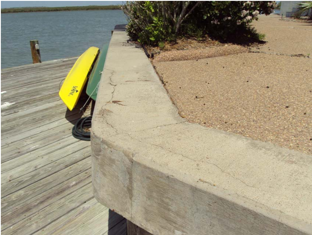
9. Lot 3, Block 3 – Settlement and Void below Concrete (4 - Poor)
