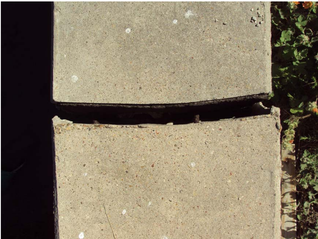
10. Lot 22, Block 3 – Cap Joint Material missing and Large Sinkhole behind Bulkhead (4 - Poor)
