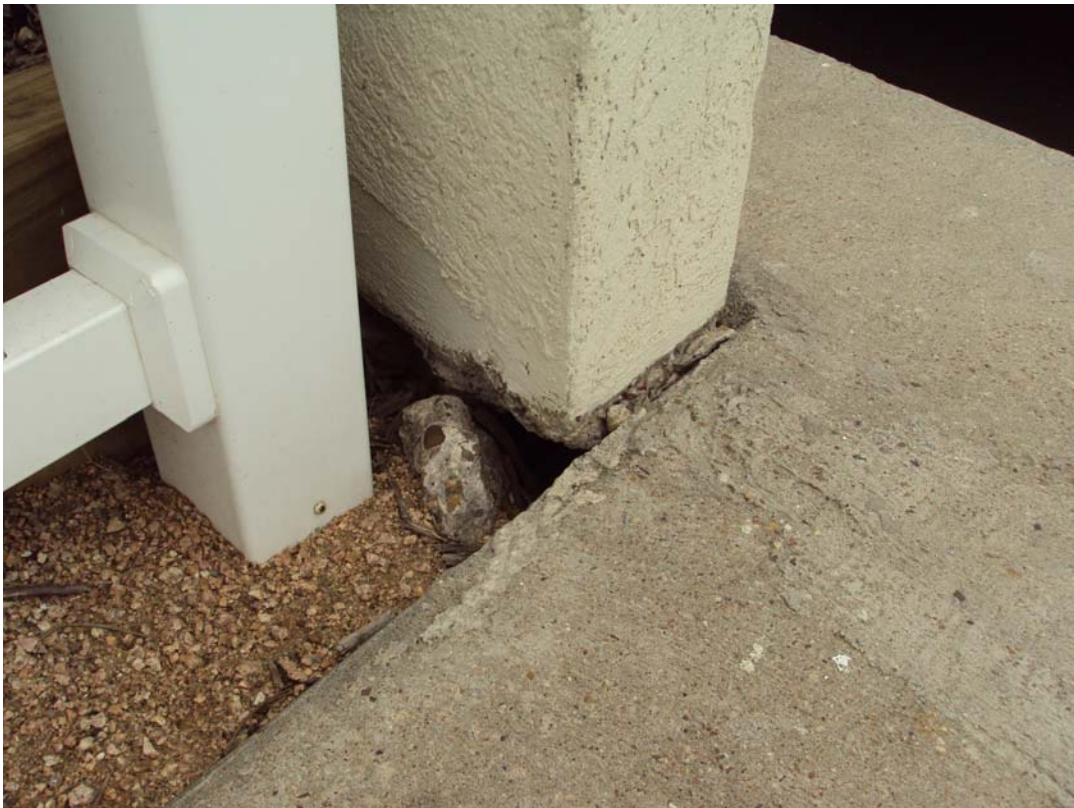
6. Lot 2, Block 1 – Small Sinkhole at Corner (3 - Fair)
