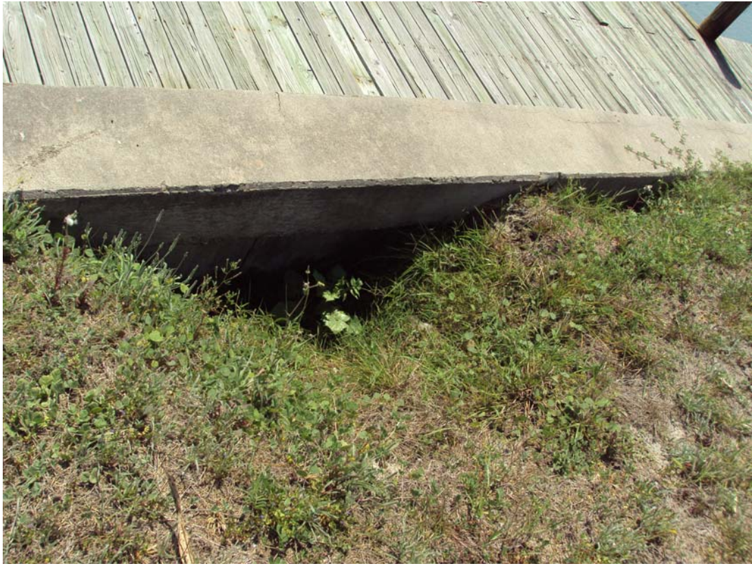
13. Lot 1, Block 2 – Large Sinkhole (4 - Poor)
