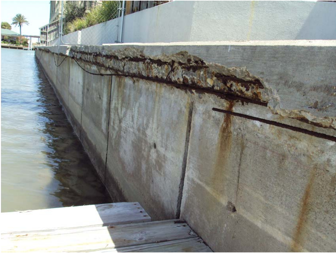
7. Lot 4, Block 3 – Major Cap Damage (4 - Poor)
