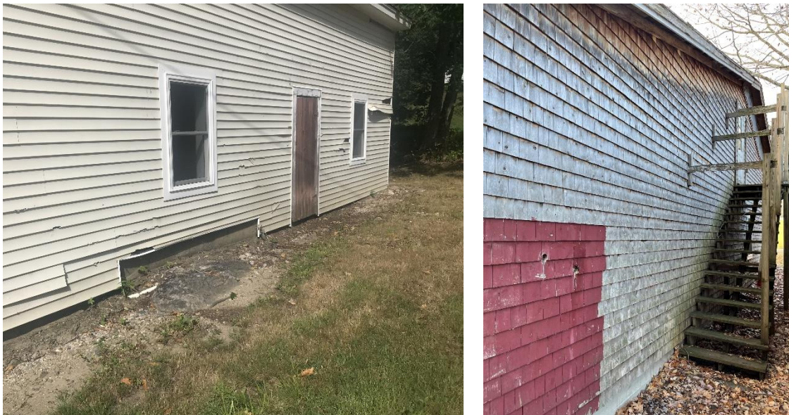
North Baldwin Fire Station generally deteriorated condition
