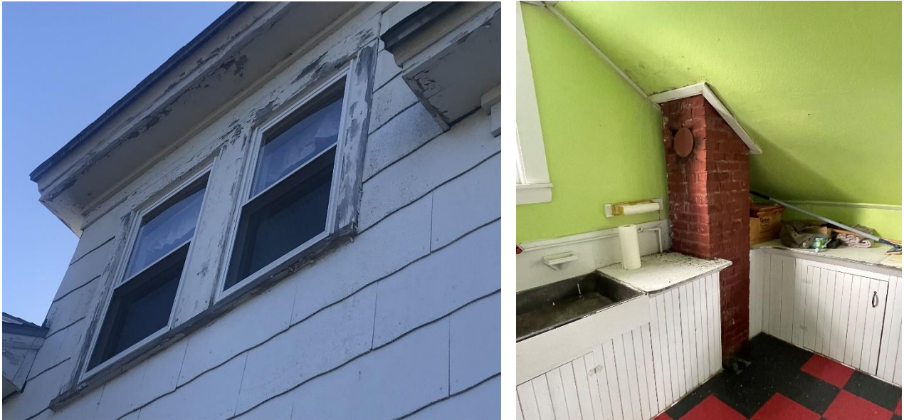
West Baldwin Fire Station generally deteriorated condition
