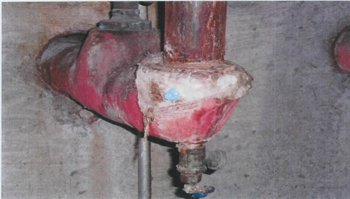
Boiler Room—An additional sample of the red pipe wrap was also collected from the shut-off valves. The sample collected tested negative for asbestos.
