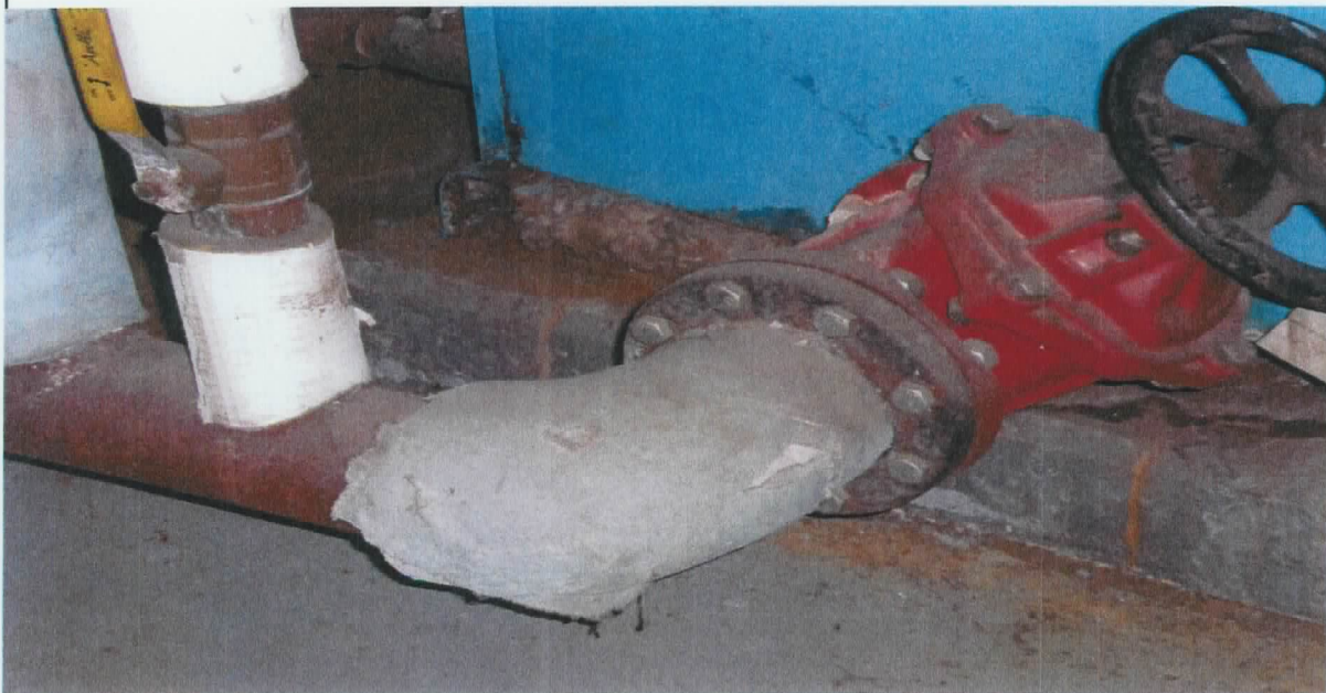
Boiler Room—A sample was collected from the green pipe wrap also attached to the boiler in the Boiler Room. The sample collected tested negative for asbestos.
