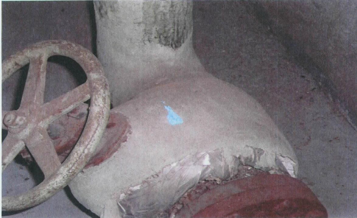
Boiler Room—An additional example of green pipe wrap was collected near the stairs. The sample collected tested negative for asbestos.
