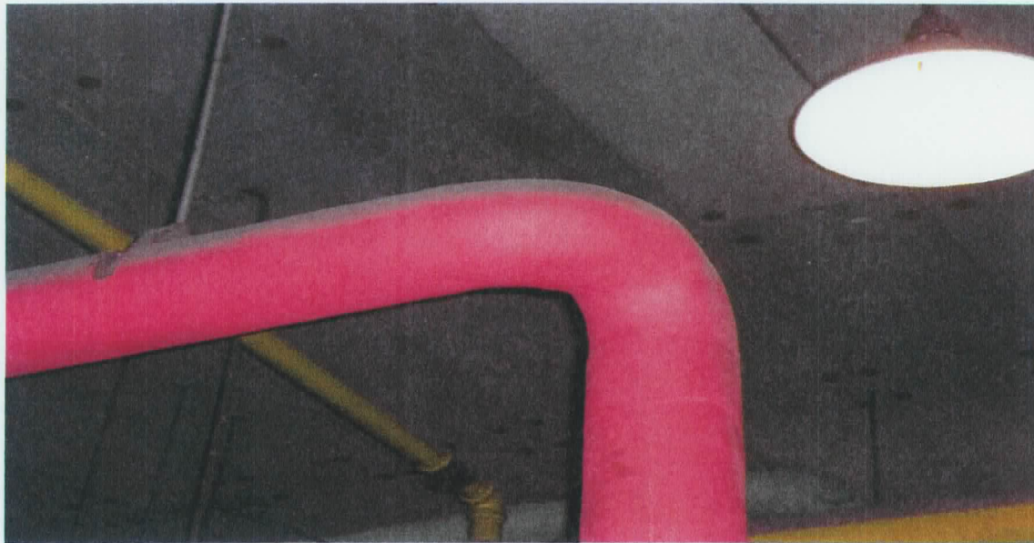
Boiler Room— A sample was collected from the red pipe wrap also connected to the boiler. The sample collected tested negative for asbestos.
