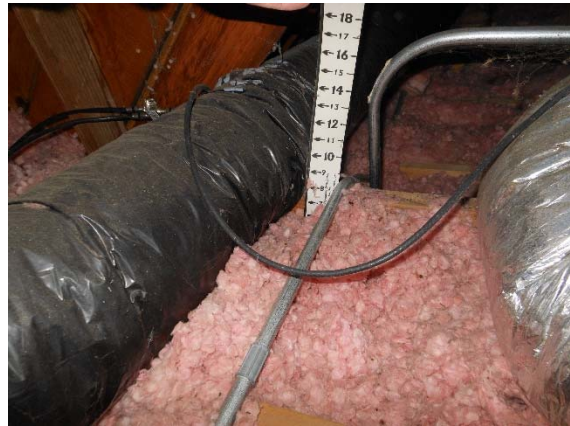
Inadequate insulation levels throughout
