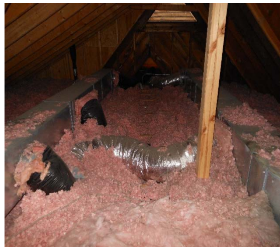
Wrapping HVAC trunk lines will reduce energy loss into attic air
