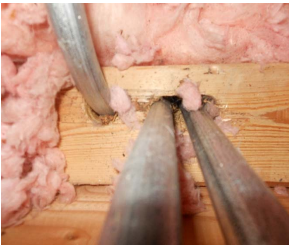
Attic leakage through pipe penetrations
