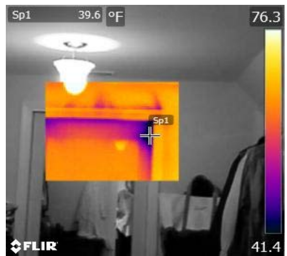
Attic leakage through master closet door
