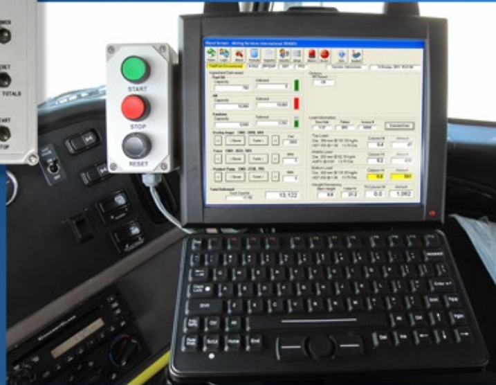
EC200 Control Panel
