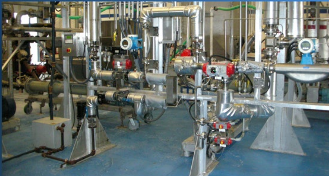
Emulsion Plant Control System
