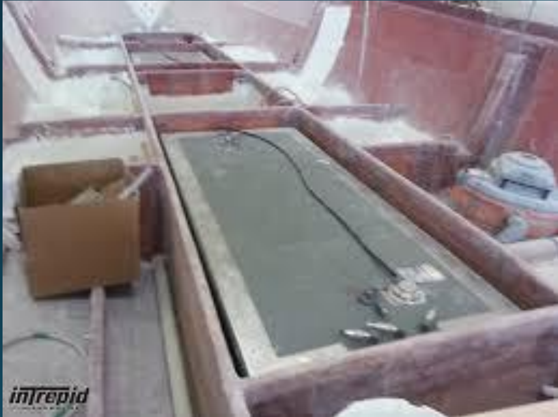
Foaming in fuel, waste and water tanks
