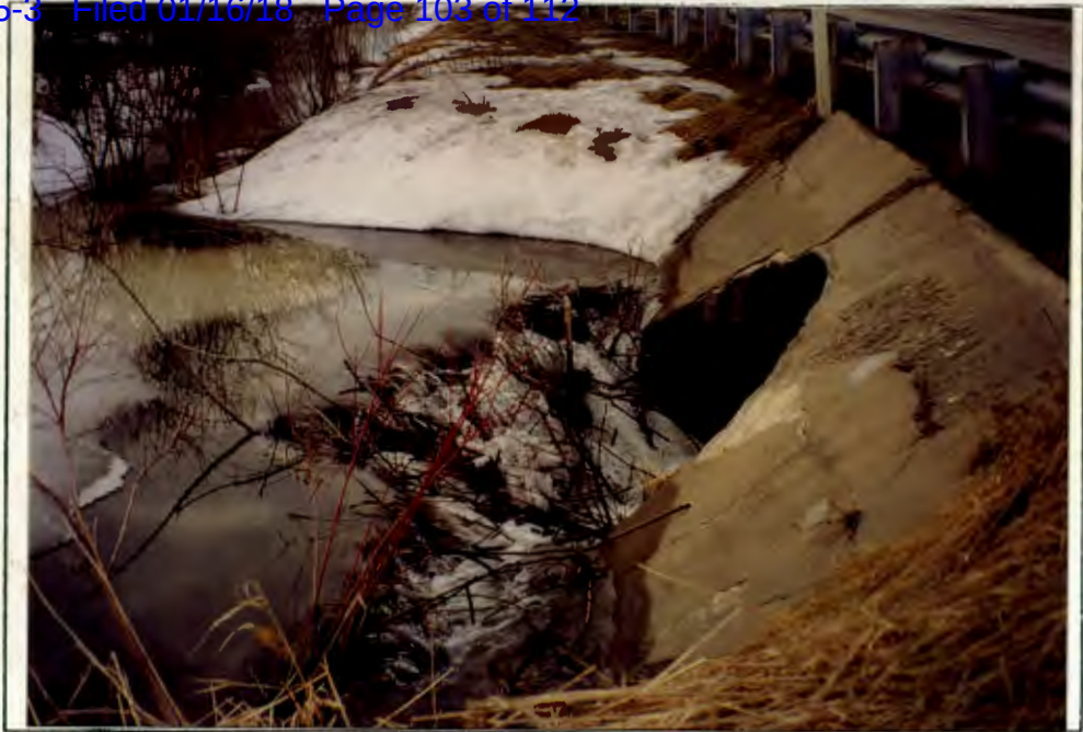
BEAVER DAM BLOCKING INLET
